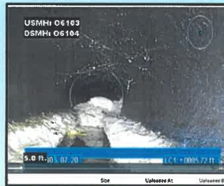
CAWD Pipe with FOG Buildup
