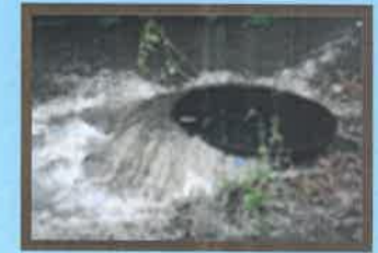
Overflow from Manhole Cover
