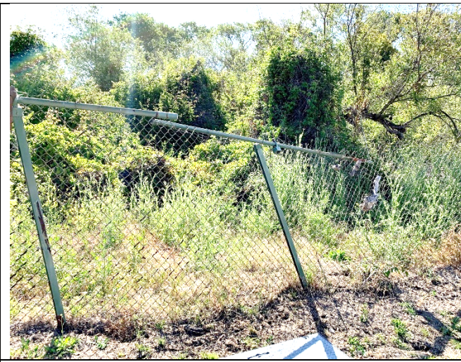
Photo: Existing Dilapidated Fence
