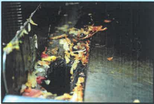
Grease Trap at a Restaurant
