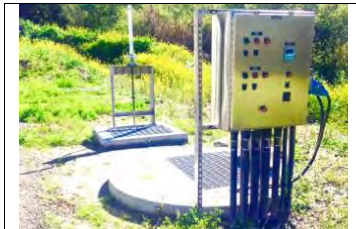
Photo: WWTP Stormwater Pump Station
