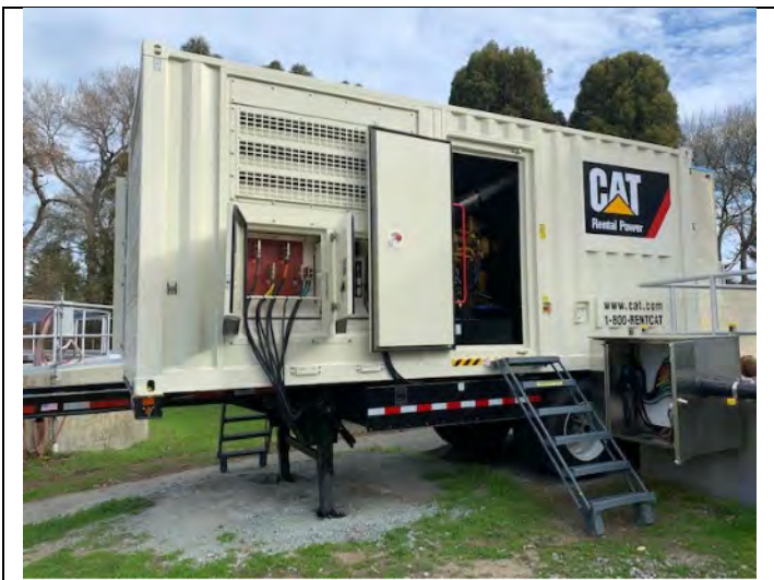
Photo: New Standby Generator
