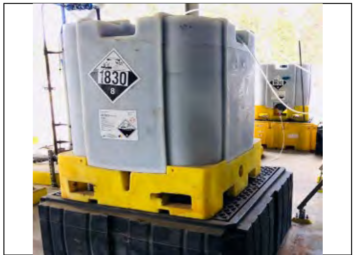
Photo: Existing totes used for Sulfuric Acid storage and Feed
