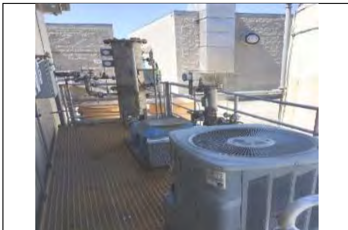
Photo: Existing Gas Conditioning System
