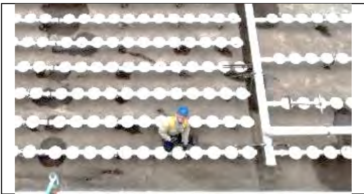
Photo: Existing air diffuser system
