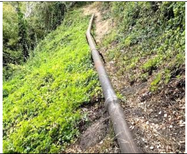
Photo: Sagged Pipeline
