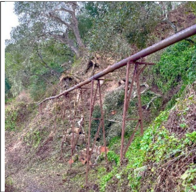
Photo: Aerial gravity pipe in easement
