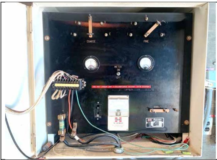
Photo: Impressed Current Rectifier
