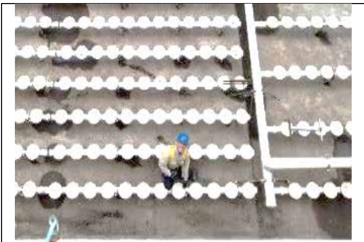
Photo: Existing air diffuser system
