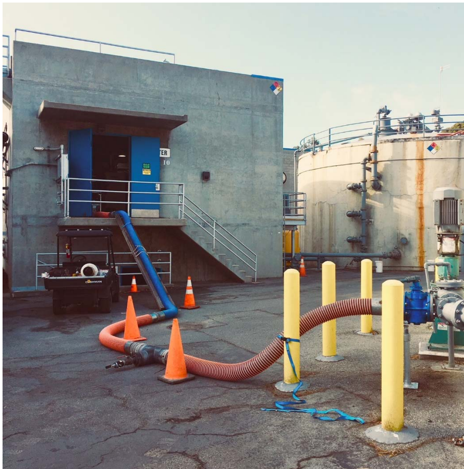
Photo 1: CAWD Temporary Transfer System
