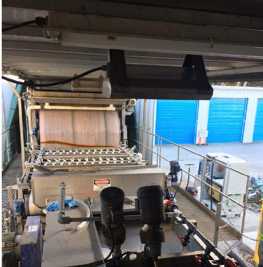
Photo 5: Mobile Dewatering Unit
