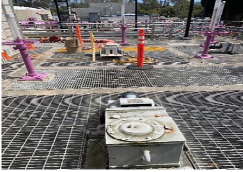
Photo: Existing Coagulation/Flocculation System and Sand Filters
