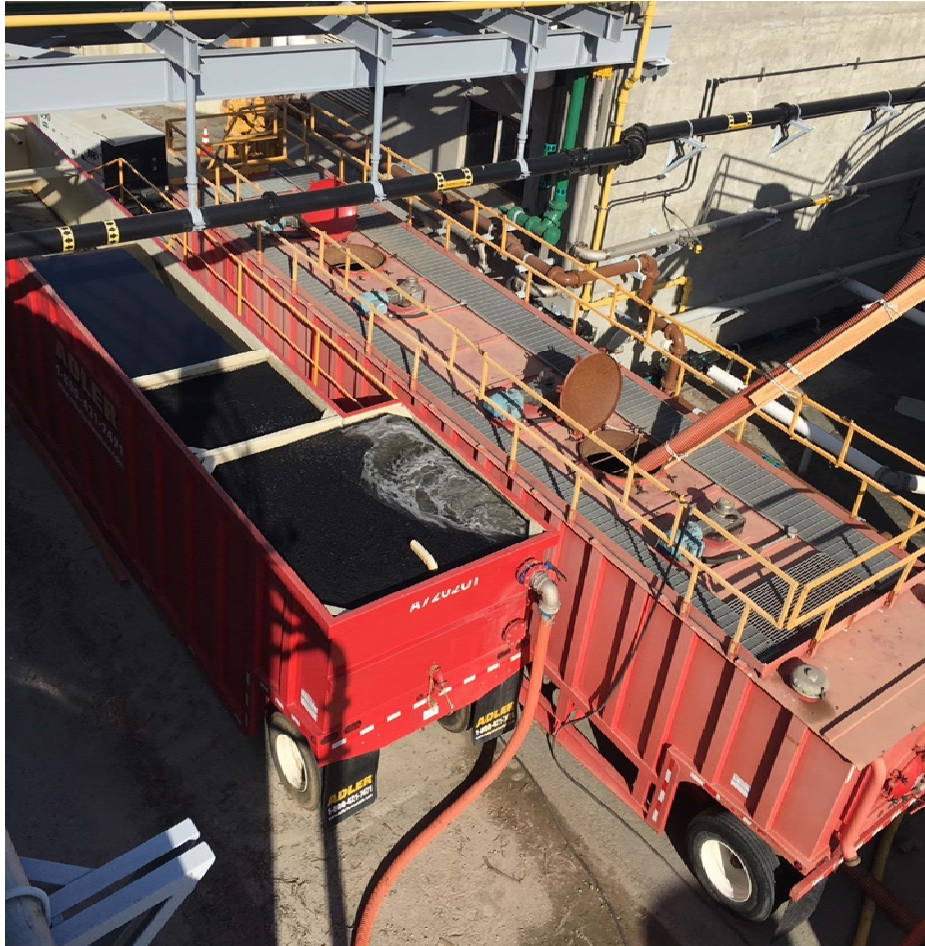
Photo 4: Mobile Dewatering Tanks
