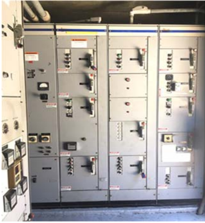
Photo: Existing Headworks Motor Control Center to Be Replaced in Project
