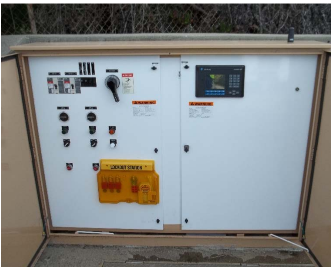
Photo: Pump station Control Panel- PLC and Operator Interface will be upgraded at Pump stations.
