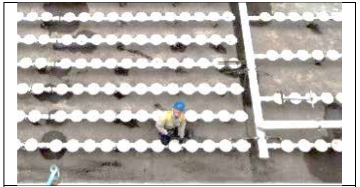
Photo: Existing air diffuser system
