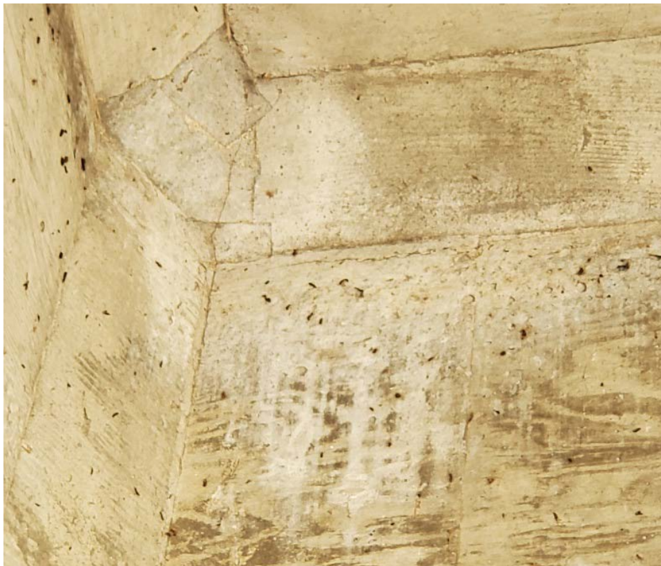
Photograph 4. Bat sign on the underside of the bridge at Valley Greens Drive.
