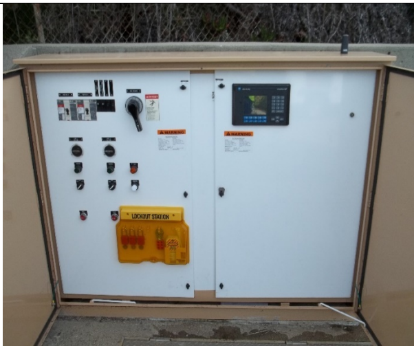
Photo: Pump station Control Panel- PLC and Operator Interface will be upgraded at Pump stations.
