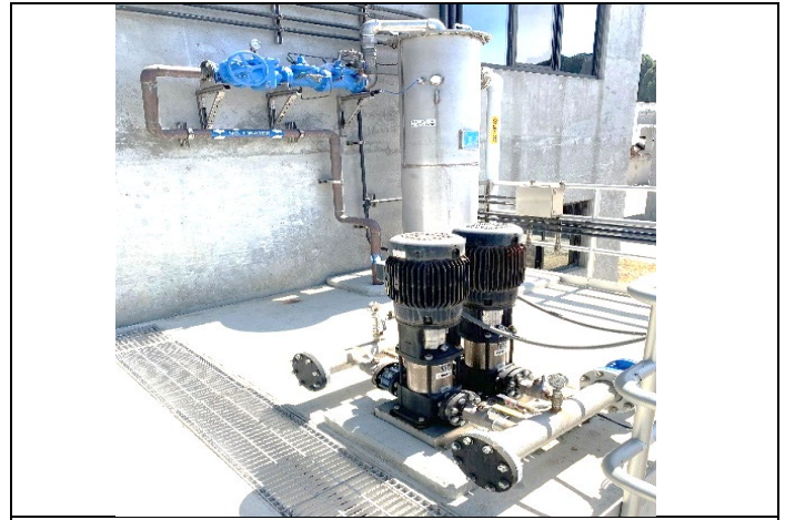
Photo: New #1 Water System where Corrosion System Project will be Installed
