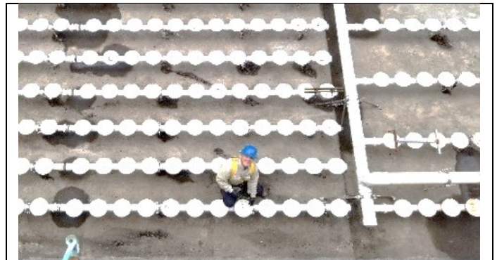
Photo: Existing air diffuser system
