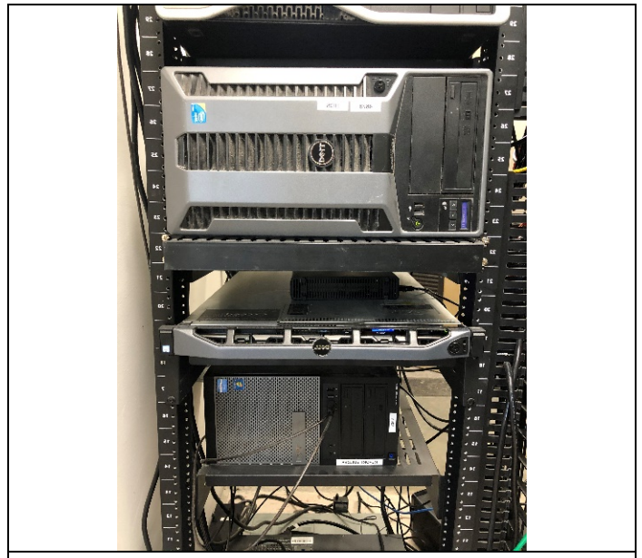
Photo: Existing Server Hardware that will be replaced in Project
