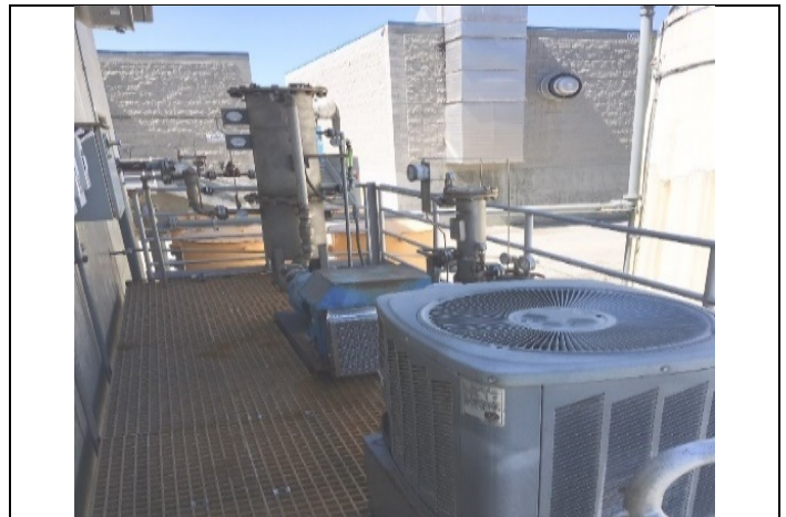
Photo: Existing Gas Conditioning System
