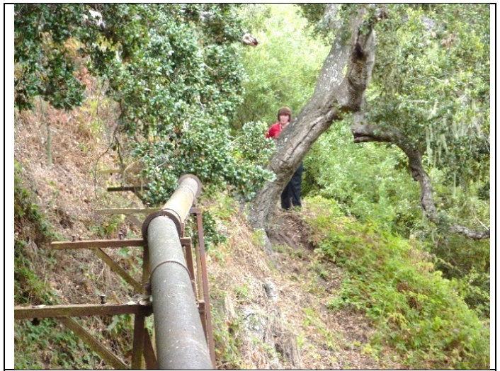
Photo: View gravity pipe in Carmel easement
