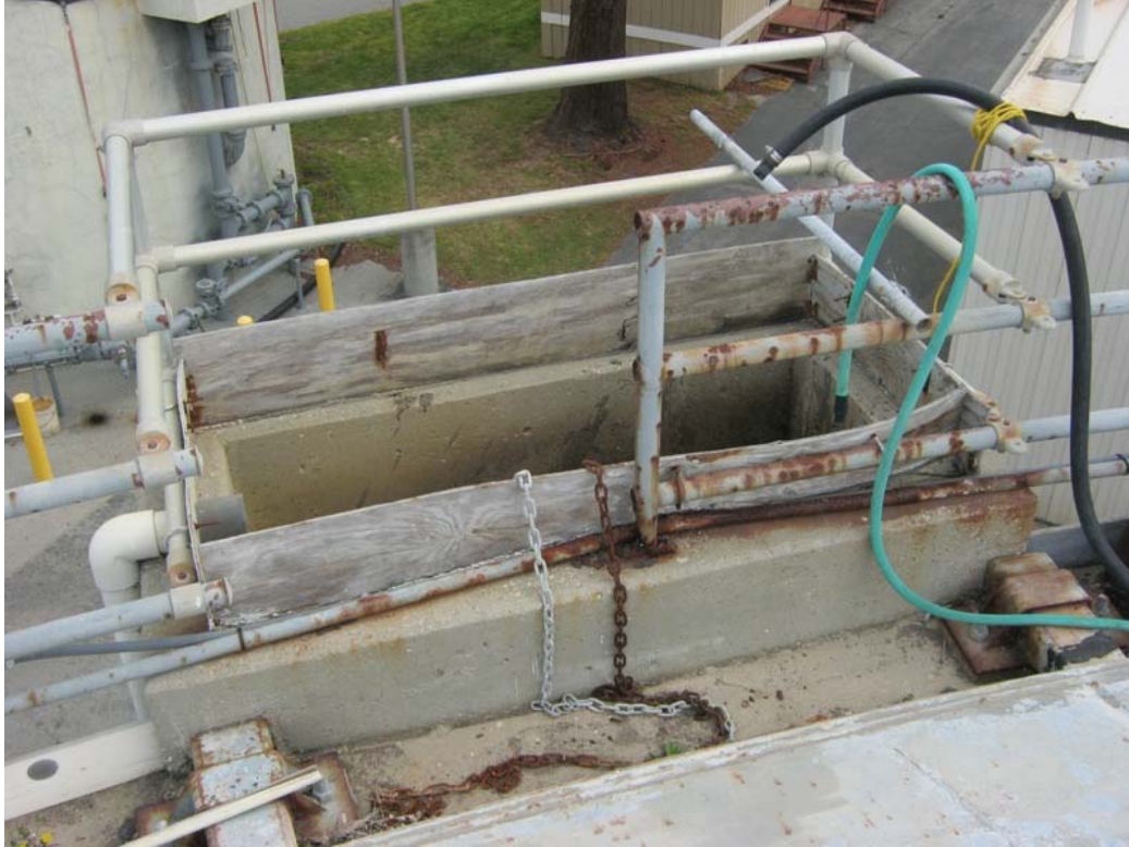
Figure 5: Rusted Roof Cover Connections
