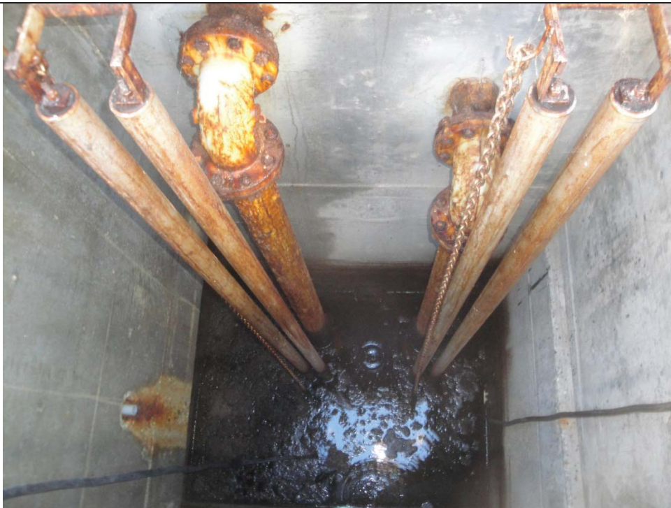
Rusted Piping and Equipment in Skimmer Pump Wet Well
