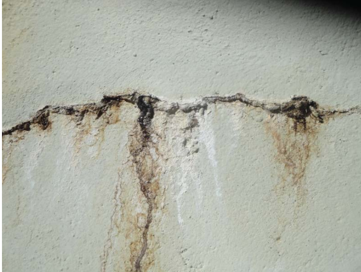
Figure 2: Minor Leakage of Sludge at the Wall Crack
