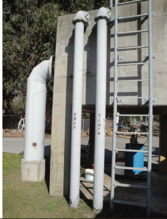
Piping Into Influent Manhole
