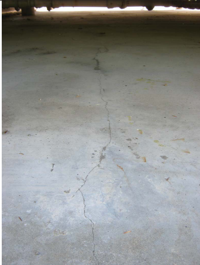
Cracks on Concrete Deck Above Chlorine Contact Channels
