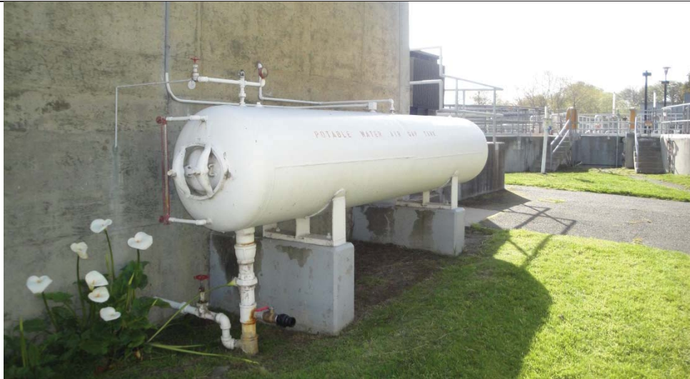
1 Water Hydropneumatic Tank
