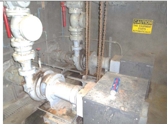
Filtrate Return Pumps
