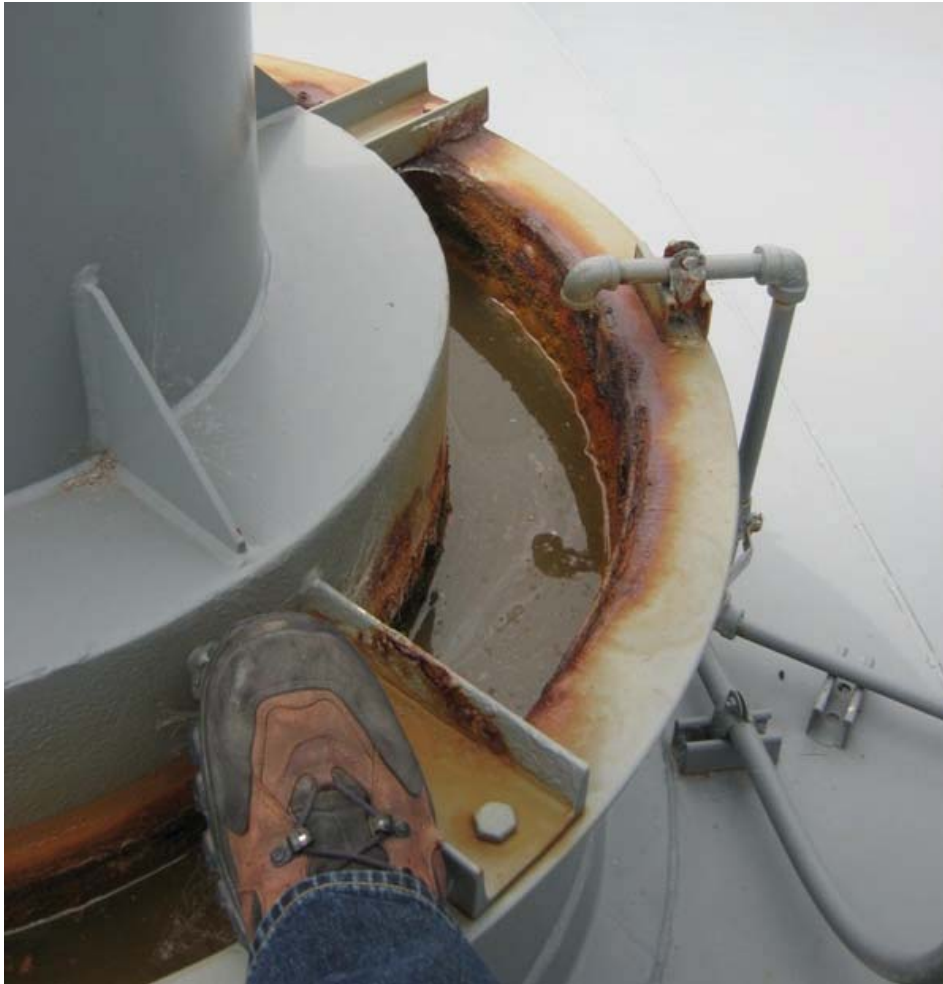
Figure 4: Rusted Water Seal on Cover
