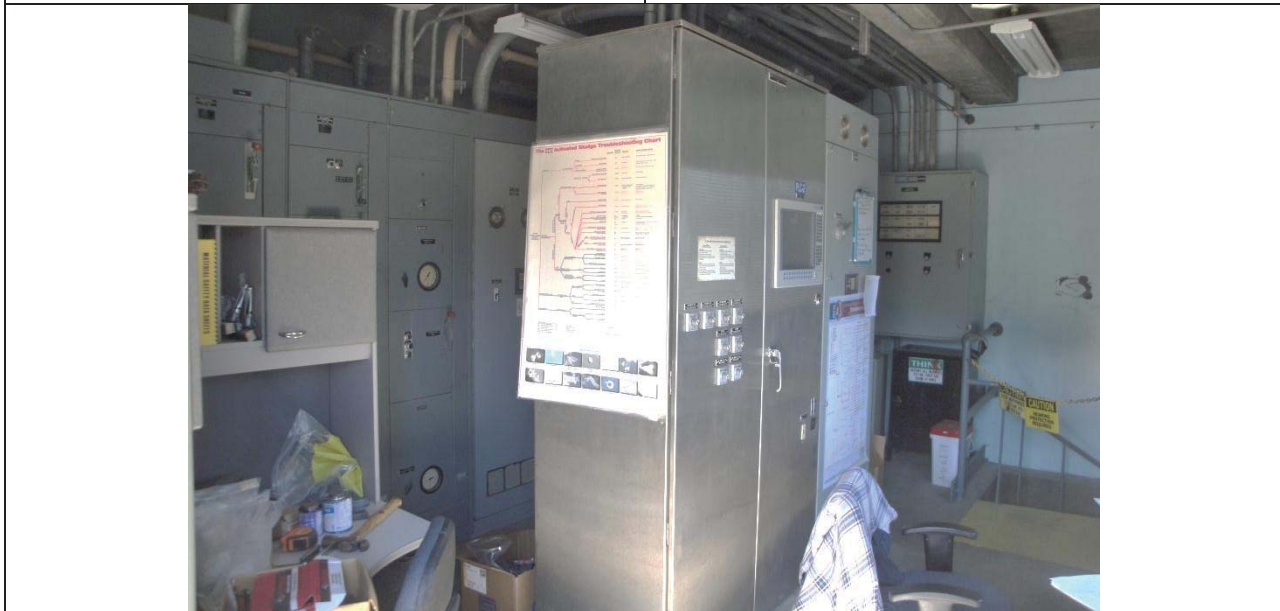
Electrical/MCC Room (Notice Desk in front of MCC)
