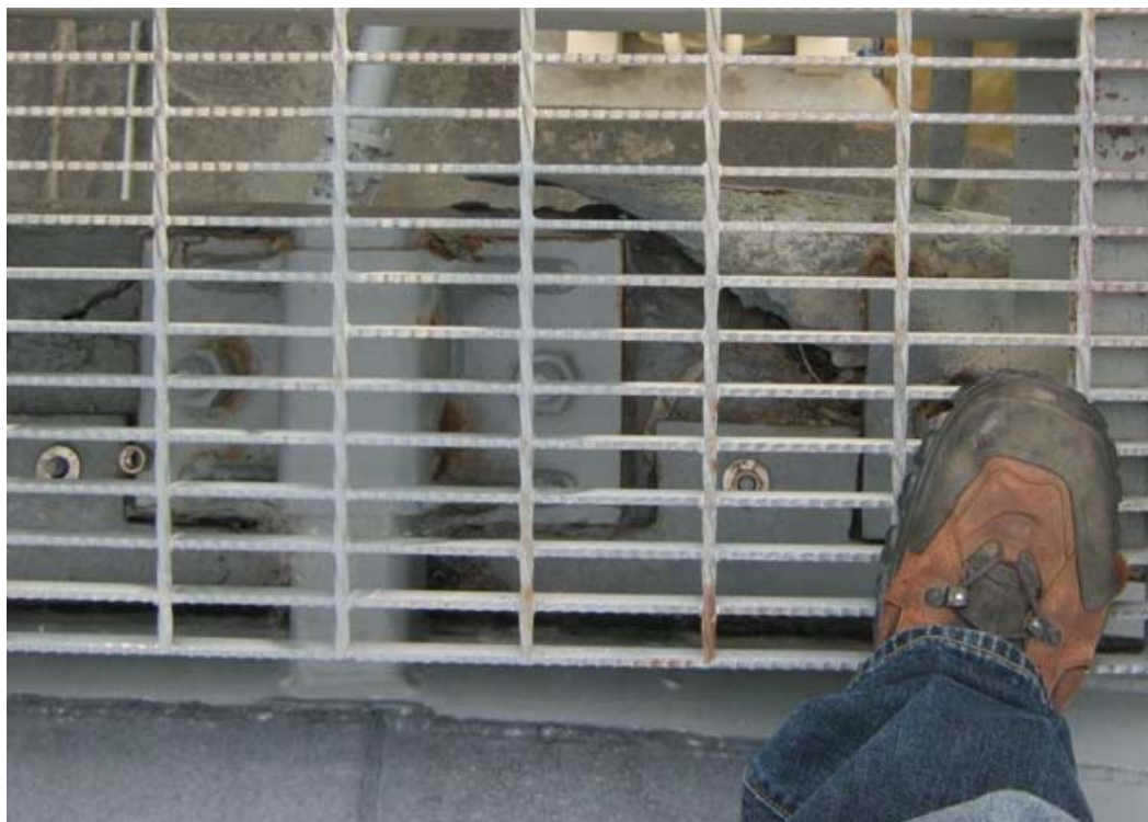
Figure 7: Cracked Concrete at Walkway Connection (Top View)
