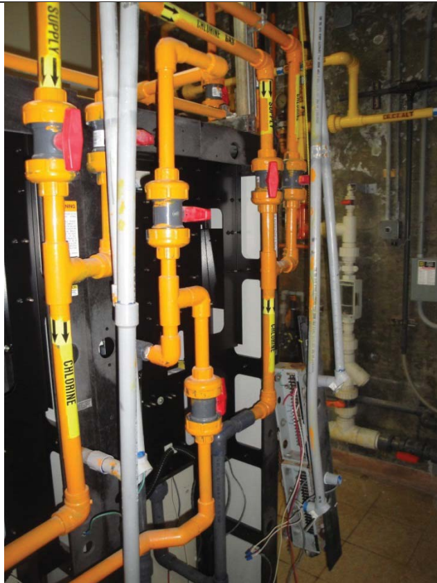
Chlorine Feed Piping
