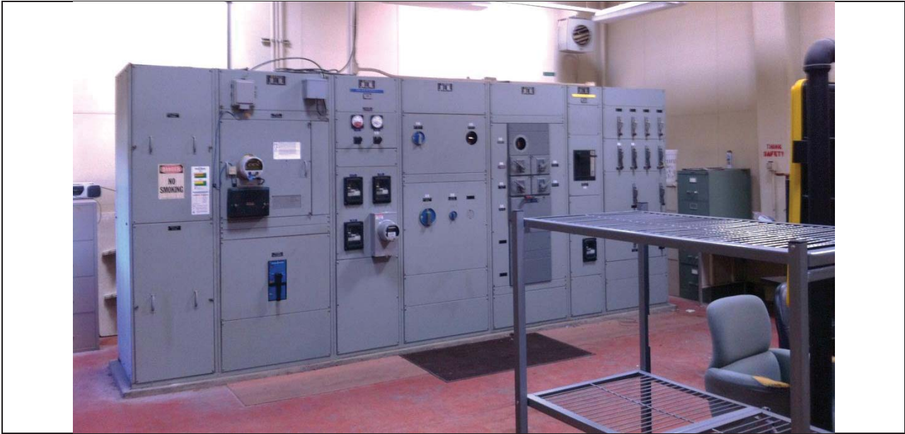
Main Power Feed Switchgear
