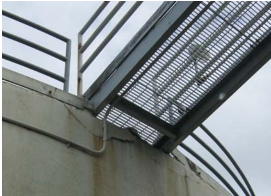
Figure 6: Spalled Concrete at Walkway Connection
