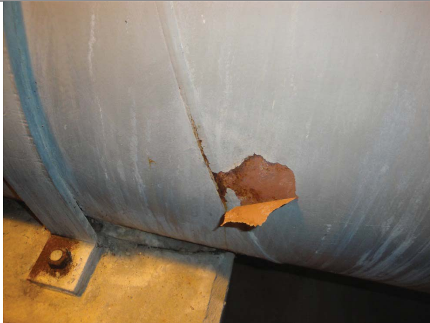
Piping in Chlorine Contact Pipe Gallery Coating Failure
