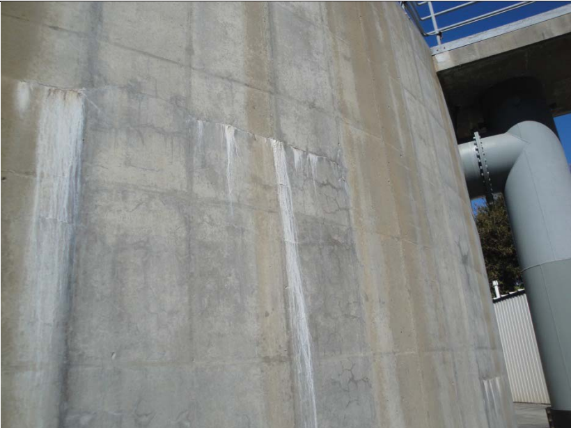
Digester 1 Concrete Horizontal Crack
