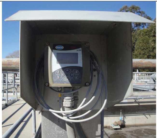
Aeration Basin Instrumentation
