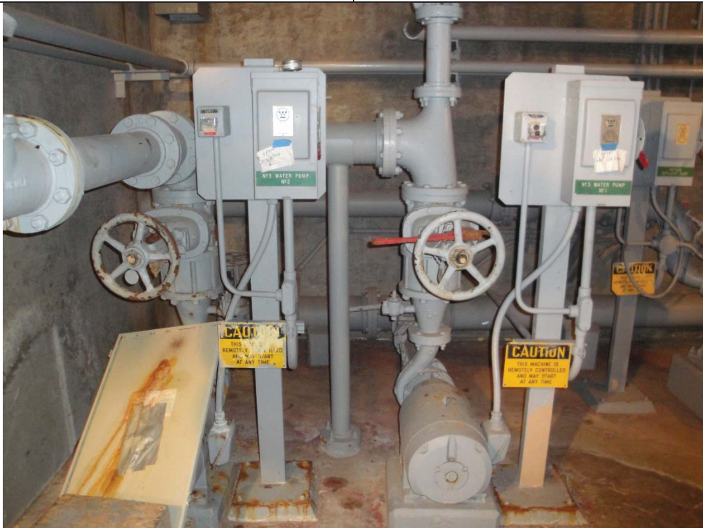
Standby 3W Pumps
