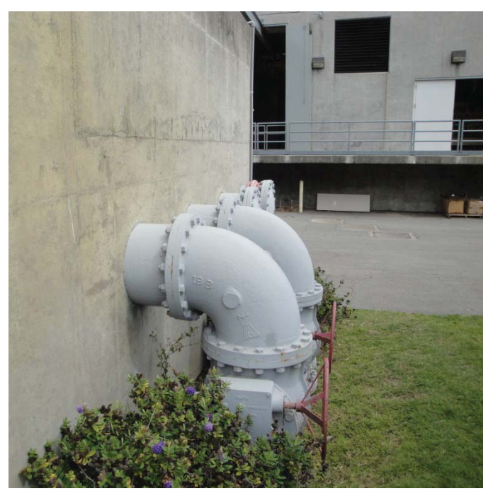
Headworks Effluent Valves
