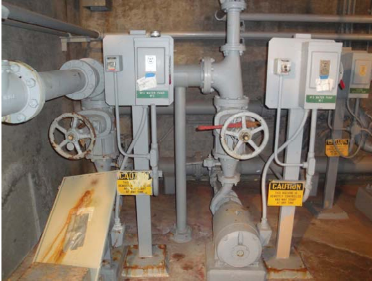
Figure 5: Treated Water (No. 3 Water) Pumps
