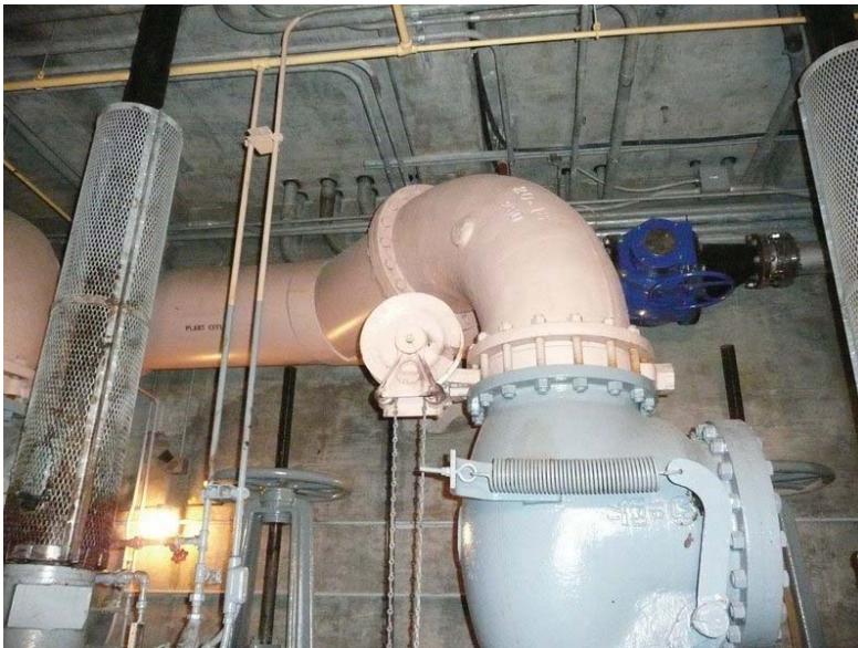
Figure 3: EPS Discharge Valves
