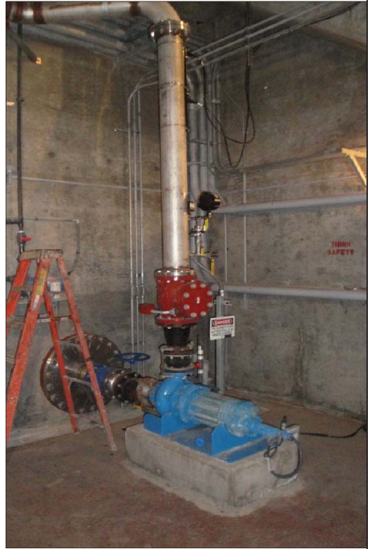
Low Flow (RO Concentrate Pump)
