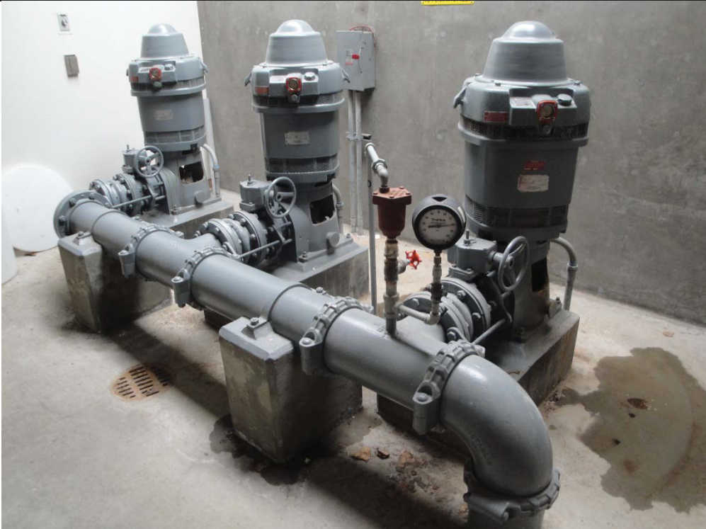
3 Water Supply Pumps
