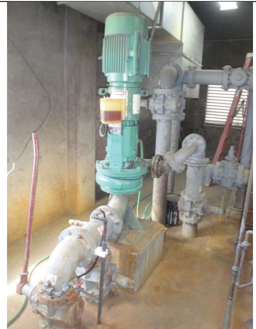
Existing Sludge Recirculation Pump – Ferric Chloride Injection Upstream
