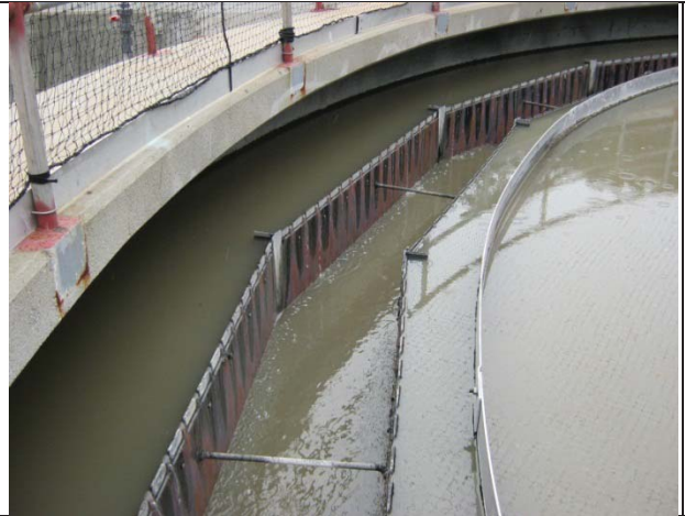
Primary Clarifier Effluent Launderer
