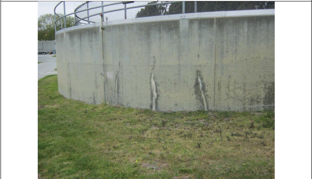
Primary Clarifier Structure with Vertical Cracks
