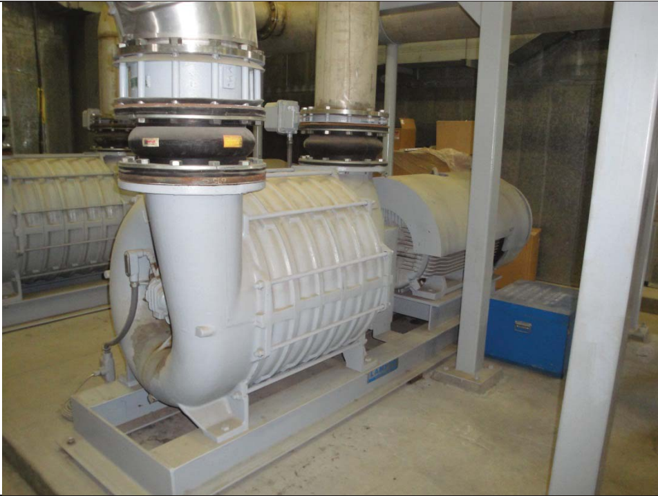
Oversized Standby Blower with Bent Shaft
