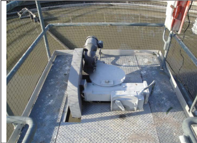
Primary Clarifier Sludge Collector Drive
