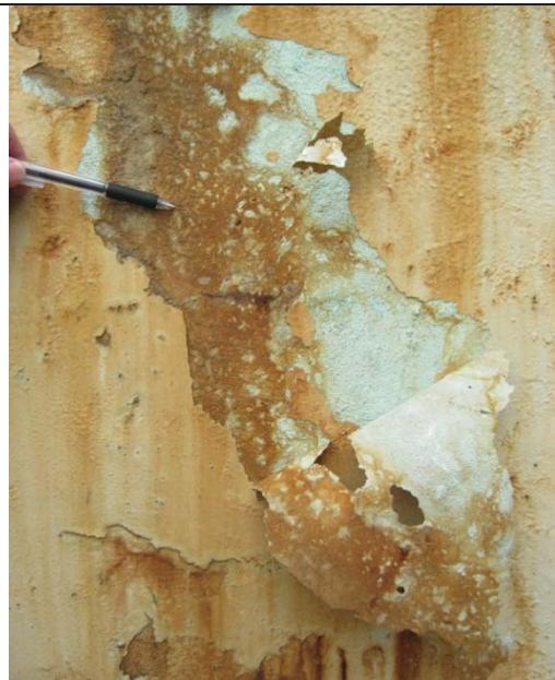
Rust staining on Digester 2 (rebar corrosion or ferric)
