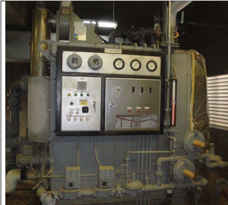
Existing Sludge Heater (Combined Boiler and Heat Exchanger)
