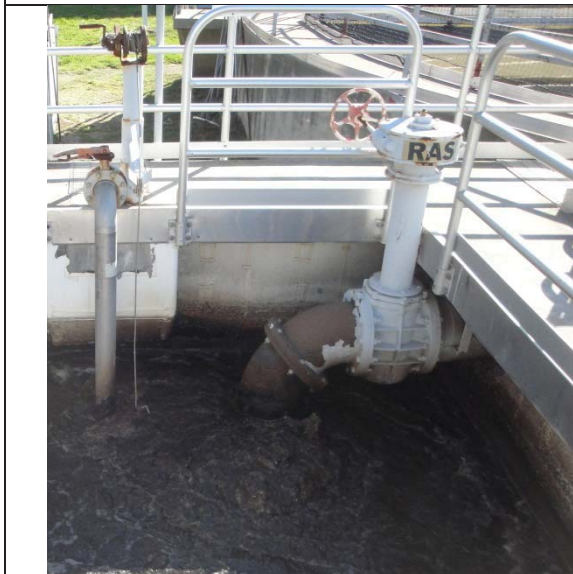
Corroded RAS Piping
