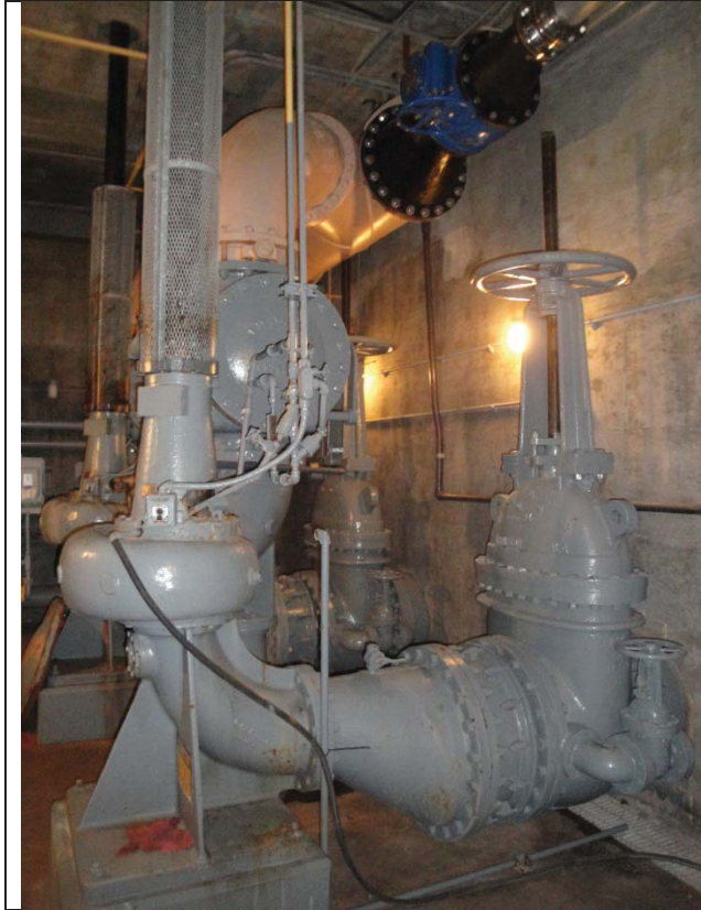
Two High Flow Effluent Pumps
