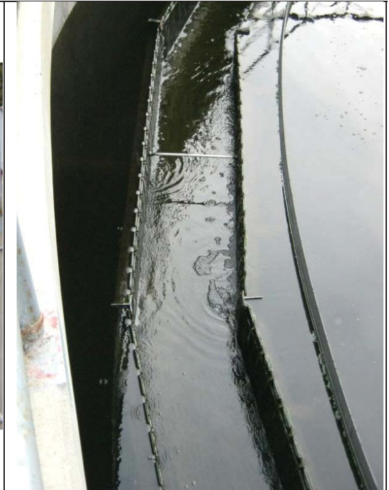
Secondary Clarifier Effluent Launderer
