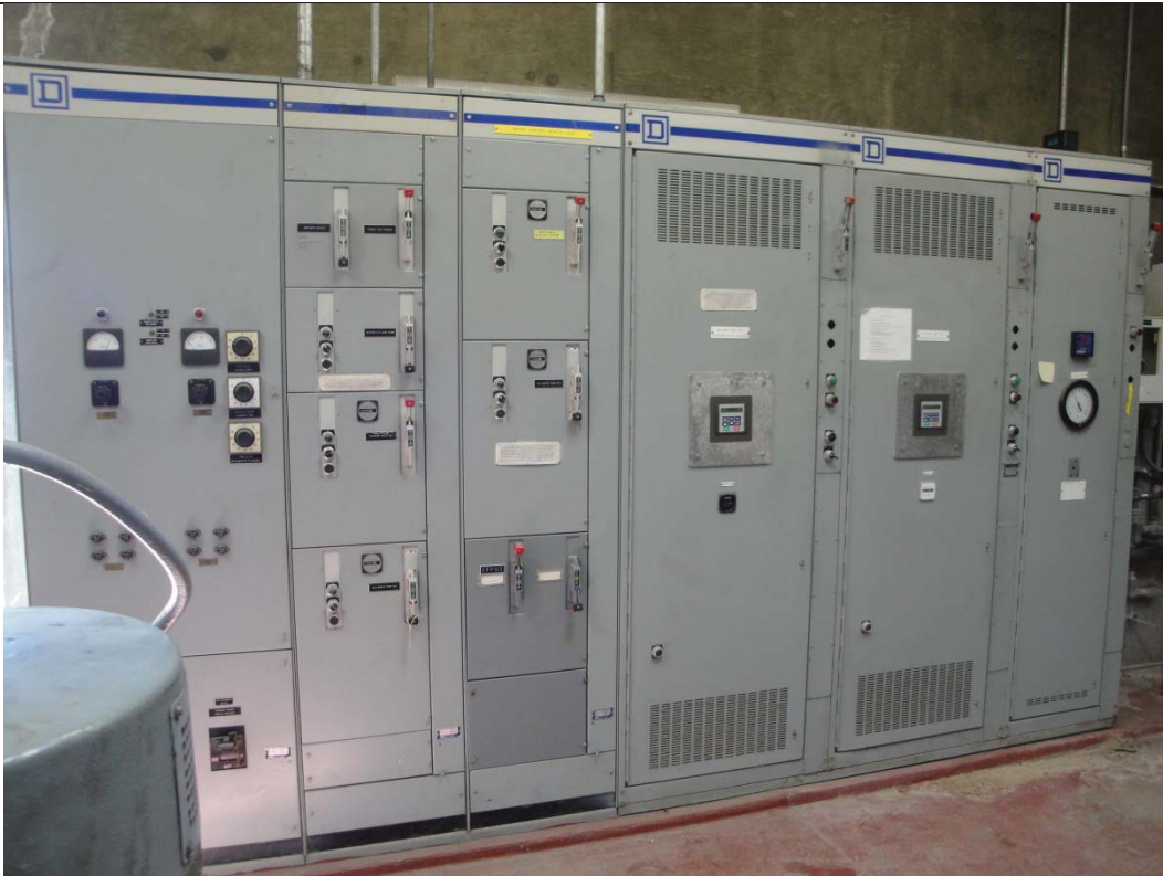
Effluent Building Electrical Gear
