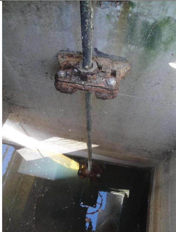
Corroded Sluice Gate Stem Operator Guide
