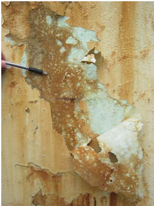
Figure 3: Rust Stain coming out from the Wall
