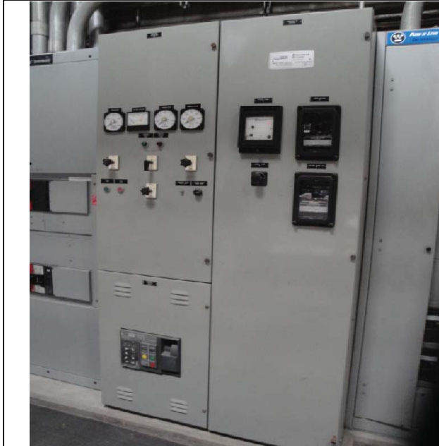
Generator Switchgear built in 1982
