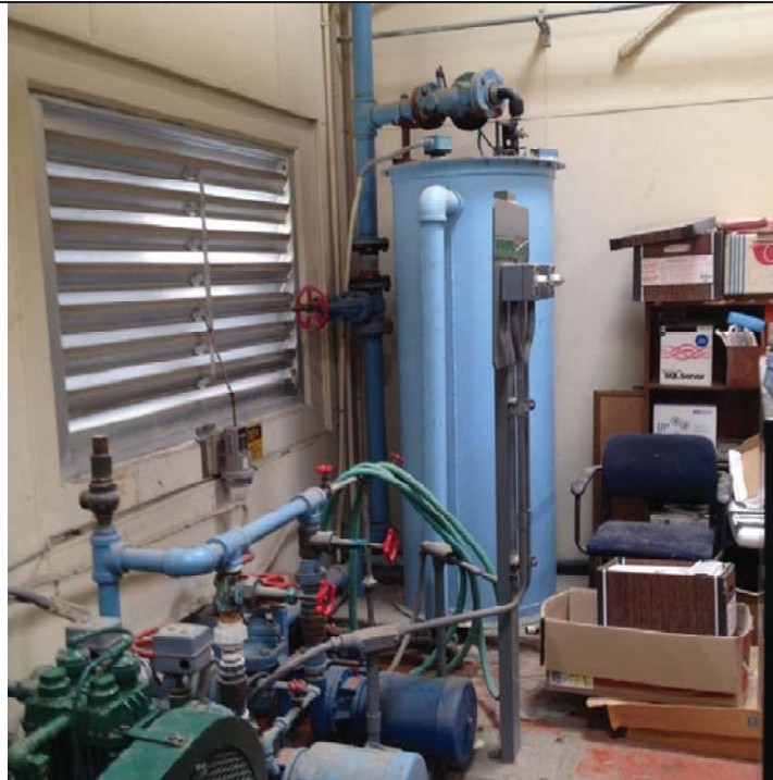
1 Water Storage Tank and Pressurization Pumps
