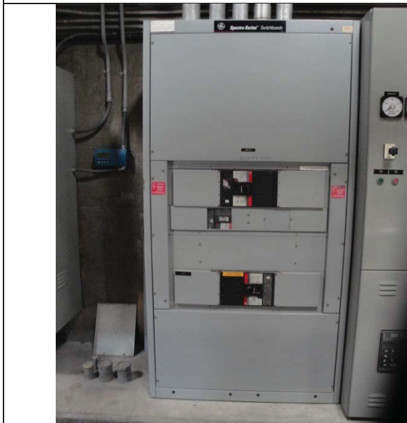
Distribution Switchboard "ISD2" (Blower Building, Main)
