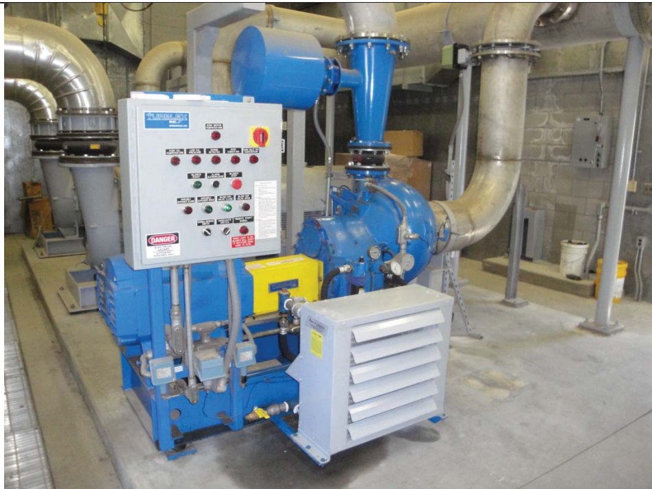
Only Reliable Aeration Blower (Turblex)
