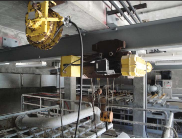
Severely Rusted Monorail Crane Equipment
