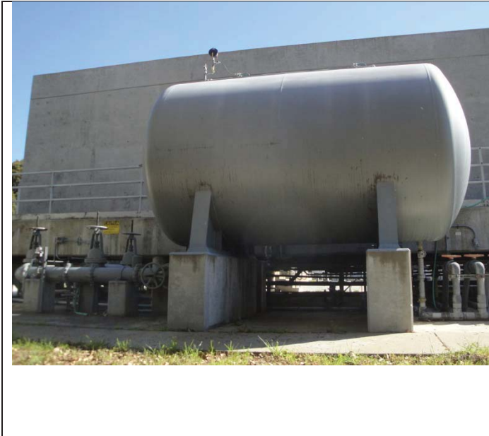
3 Water Hydropneumatic Tank
