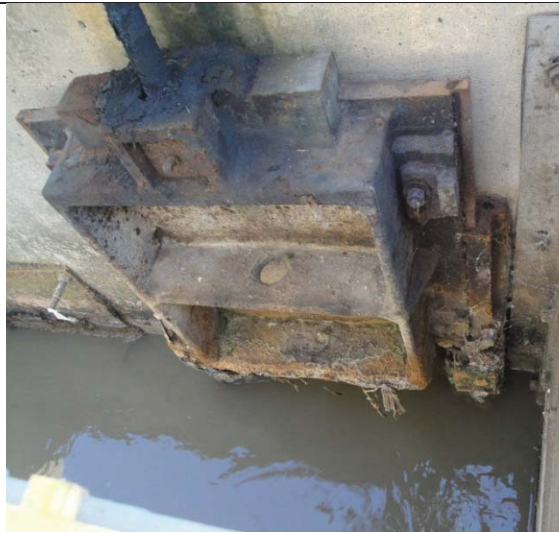
Corroded Influent Manhole Sluice Gate
