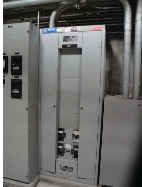
Distribution Switchboard "ISD" (Sludge Dewatering, Lab, Influent)
