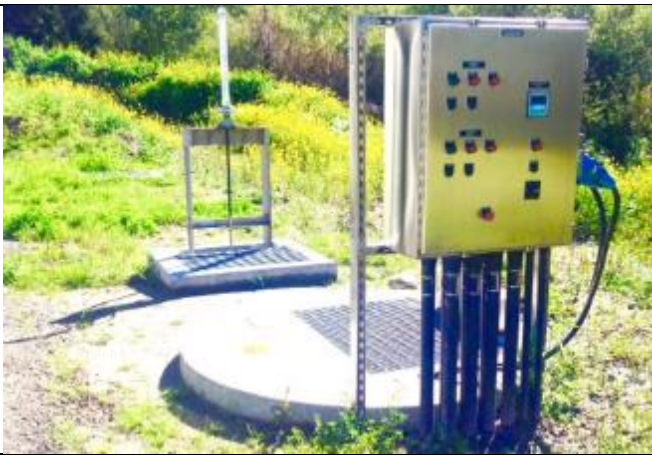
Photo: WWTP Stormwater Pump Station
