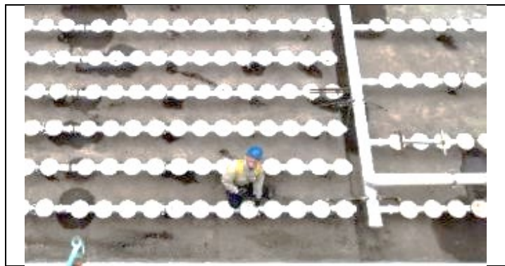
Photo: Existing air diffuser system
