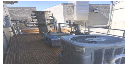
Photo: Existing Gas Conditioning System
