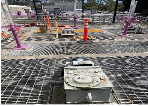
Photo: Existing Coagulation/Flocculation System and Sand Filters
