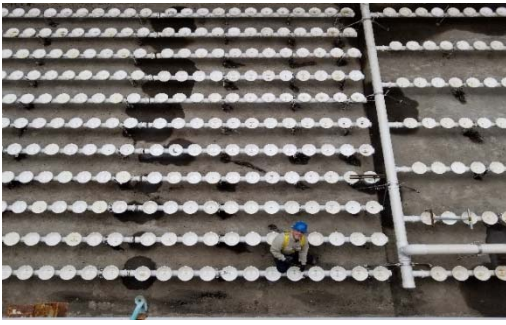
Photo: Existing air diffuser system
