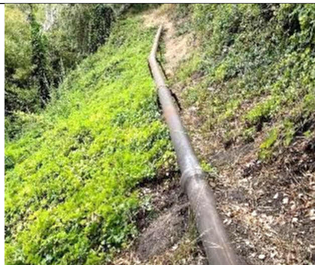
Photo: Sagged Pipeline
