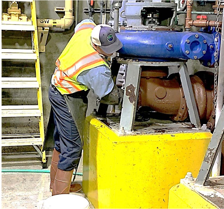
Reaching into Pump
