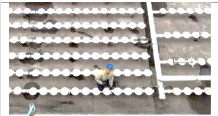
Photo: Existing air diffuser system
