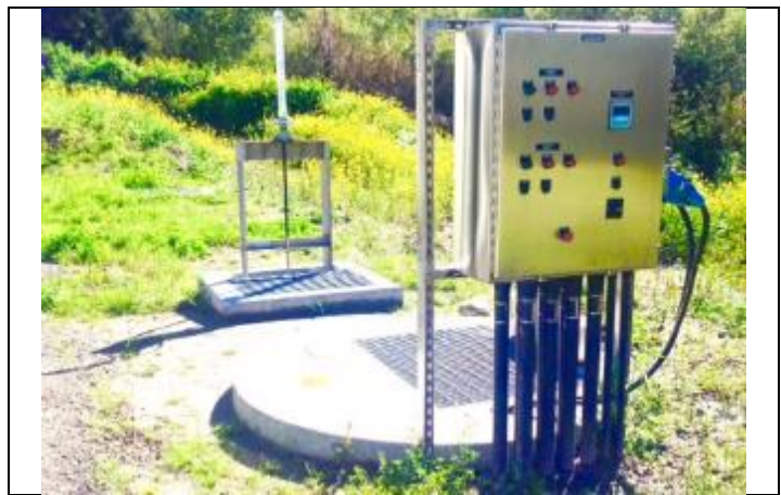
Photo: WWTP Stormwater Pump Station
