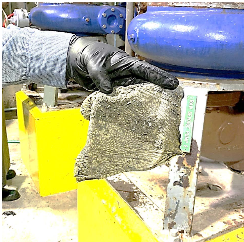
Typical Intact Wipe
