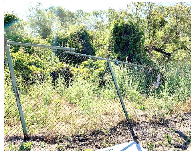
Photo: Existing Dilapidated Fence
