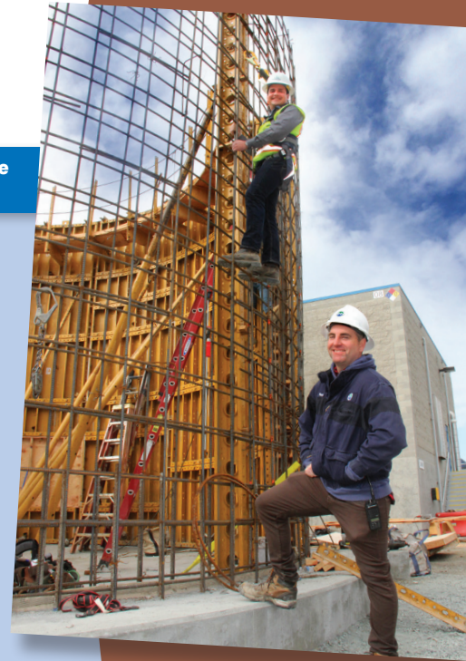
CAWD Principal Plant Engineer Patrick Treanor (foreground) and Construction Manager Evan Currie of Currie Engineers inspect progress on the plant's new sludge holding tank. The 73,000-gallon tank will meet current seismic standards, replacing our previous tank which served the community for 84 years.
