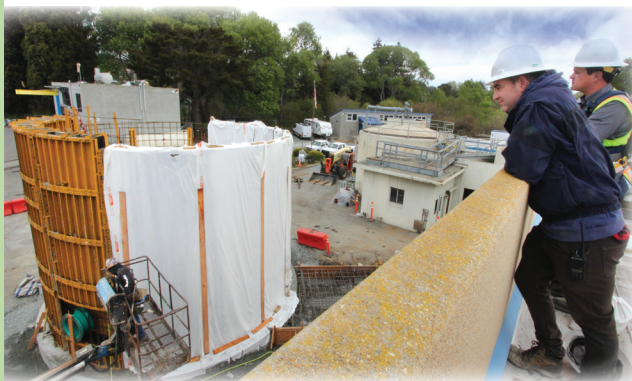
A TOPSIDE VIEW OF OUR COMMUNITY'S NEW SLUDGE HOLDING TANK CAWD's treatment plant renovation will be largely completed next year, on budget and ahead of time, to ensure public health and safety, and protect the local environment for the next 30 years.
