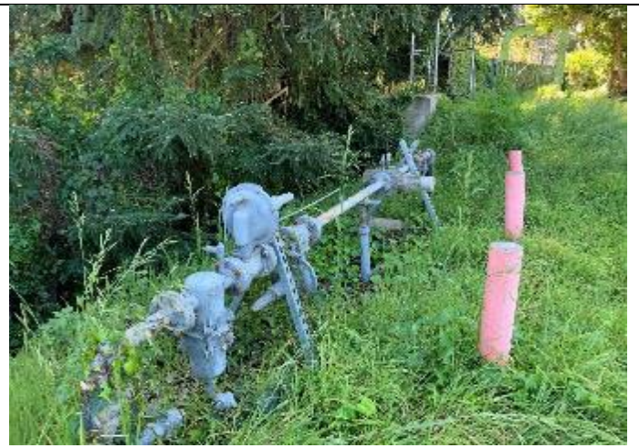
Photo: Gas Meter on North Side of River
