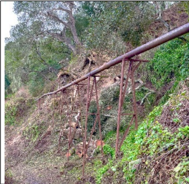
Photo: Aerial gravity pipe in easement
