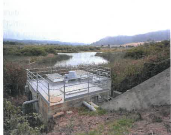
Calle la Cruz Pump Station
