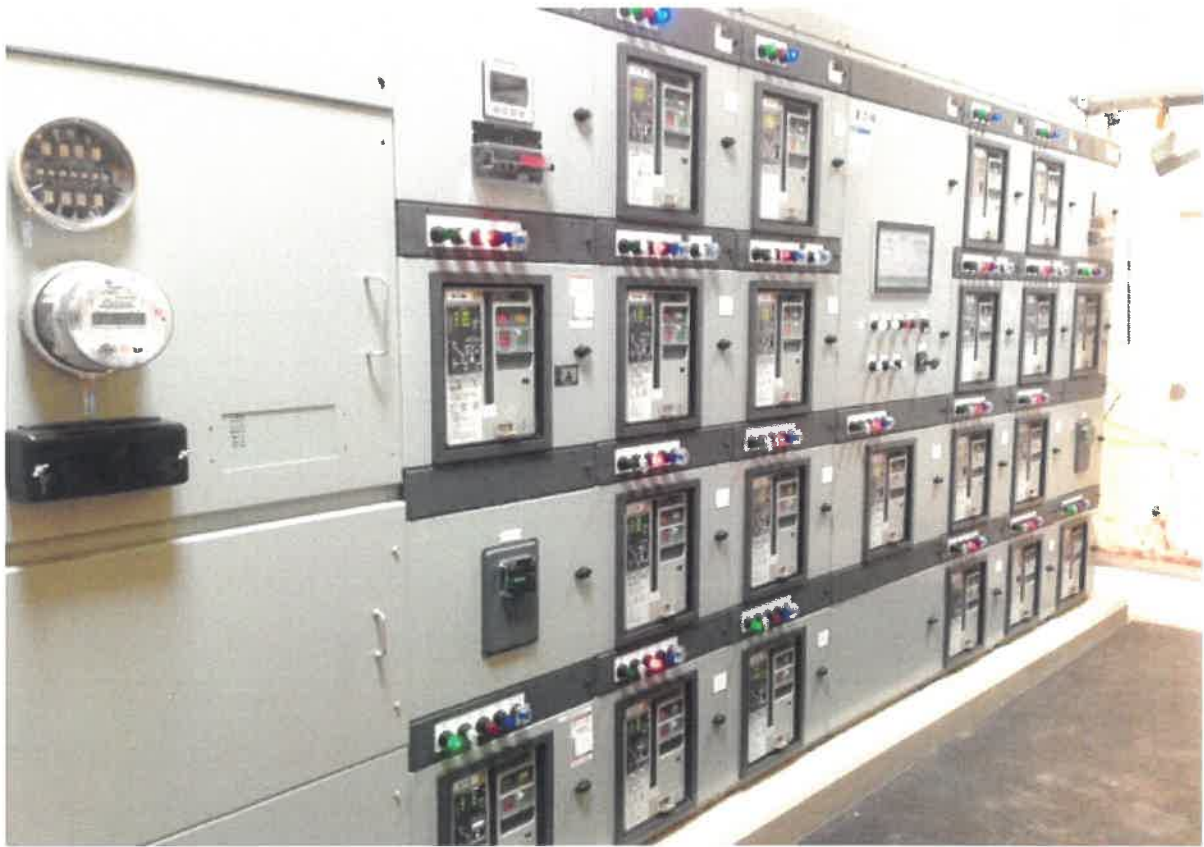
Primary Motor Control Center – installed 2017
