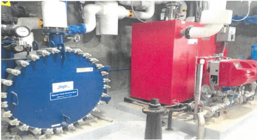
Digester Control Building #1 – Spiral Heater and Boiler
