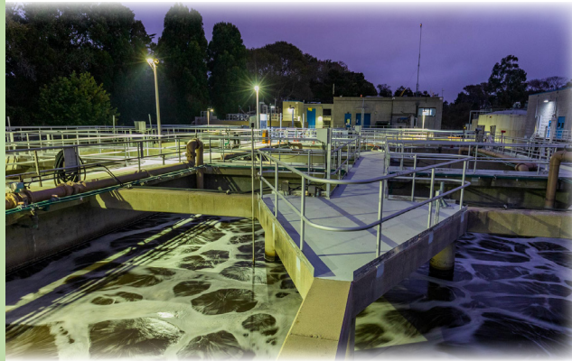
NIGHTWATCH AT THE PLANT In adherence with COVID guidelines, CAWD staff are split into day and night shifts to ensure that we have skilled plant operators even if one shift has to quarantine.
