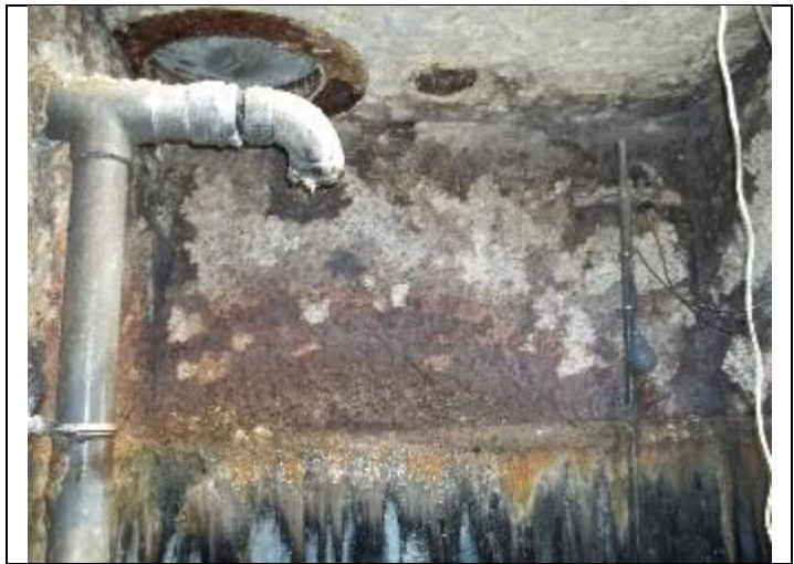
Photo: View H2S damage to Calle La Cruz wet well
