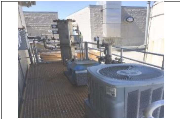
Photo: Existing Gas Conditioning System
