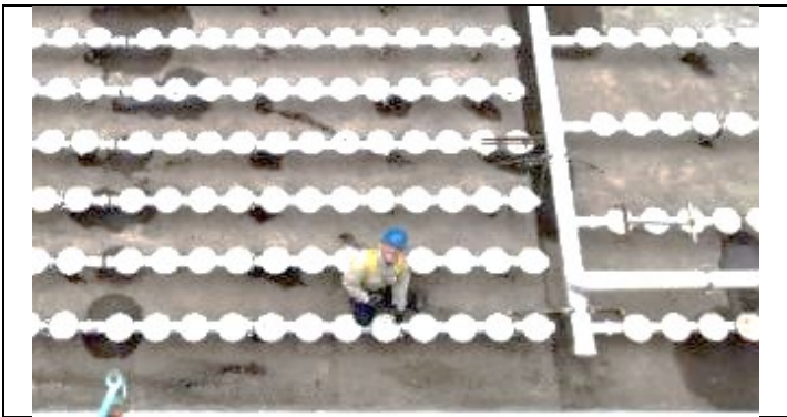
Photo: Existing air diffuser system
