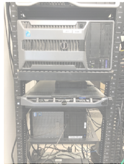
Photo: Existing Server Hardware that will be replaced in Project
