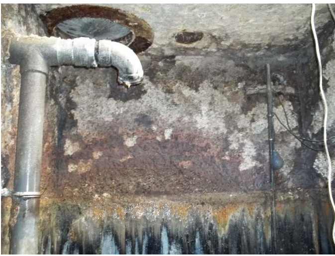
Photo: View H2S damage to Calle La Cruz wet well
