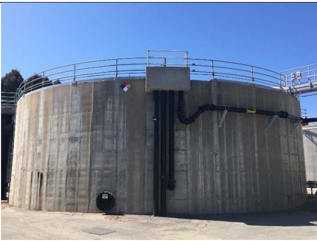
Photo: Digester No. 1
