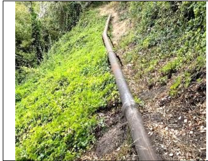
Photo: Sagged Pipeline
