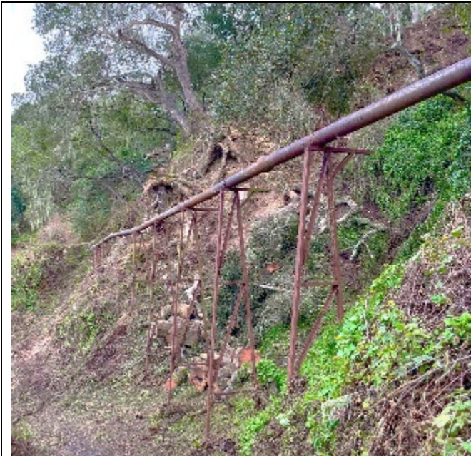
Photo: Aerial gravity pipe in easement
