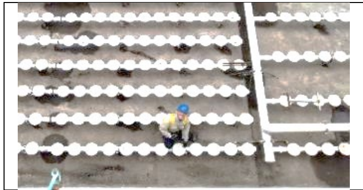
Photo: Existing air diffuser system
