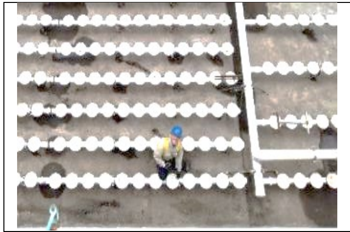
Photo: Existing air diffuser system
