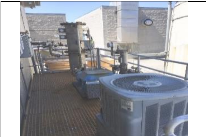
Photo: Existing Gas Conditioning System
