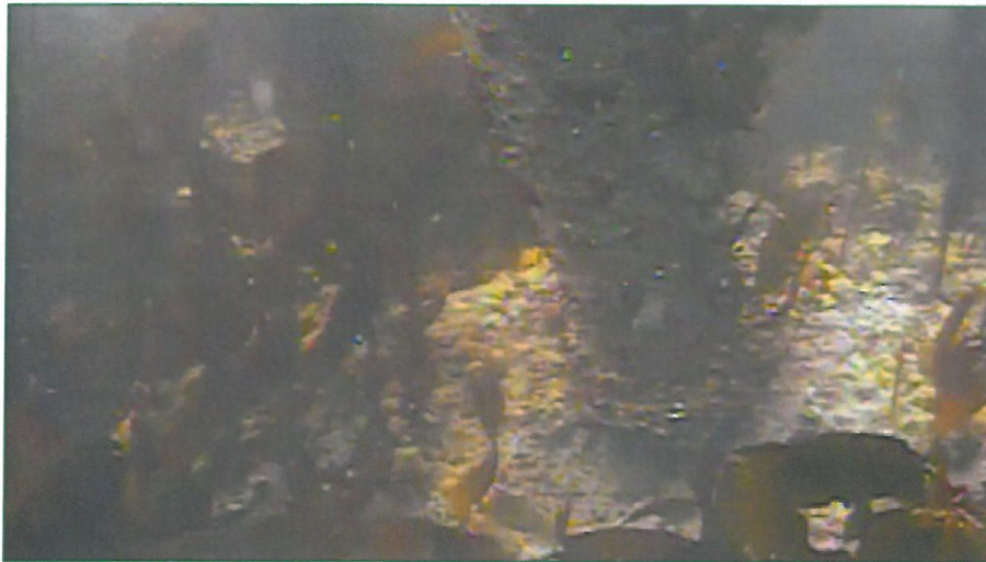
Figure 6 -- Typical view underwater of the diffuser pipe at the seabed. Typically the 24 in. pipe was not visible and appeared to be encased in either tremie concrete or hard coral.
