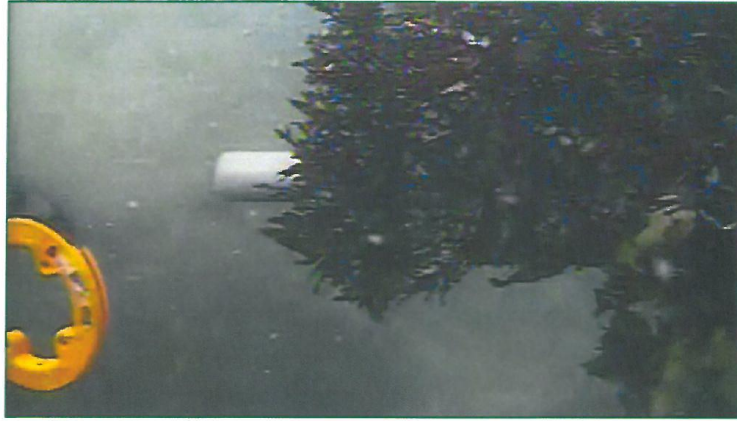
Figure 4 -- View underwater of the probe setup with an electrician's pull wire, introduced through the backflow prevention valve via a small piece of plastic pipe.
