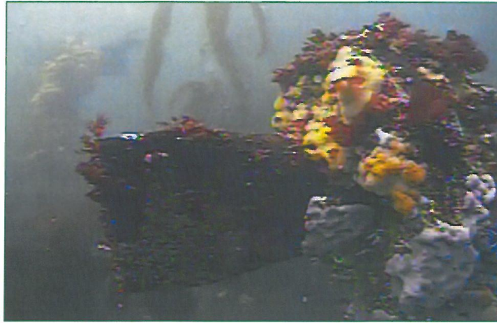
Figure 5 View underwater of a typical duckbill type backflow prevention valve and riser.
