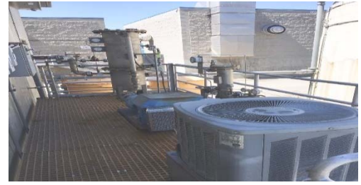
Photo: Existing Gas Conditioning System
