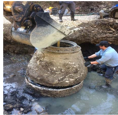
Photo: View of a temporary repair of a manhole in Hatton Canyon
