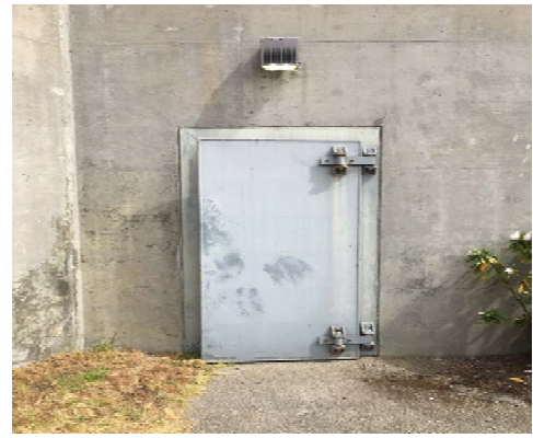
Photo: Old Flood Door in Headworks Basement
