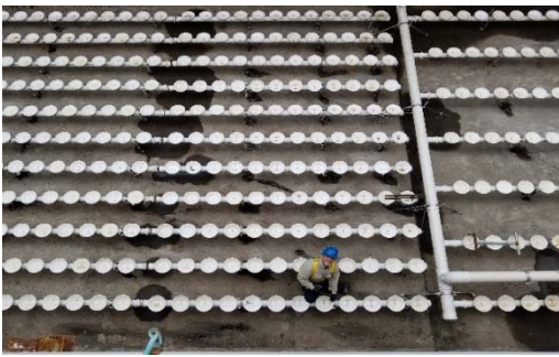
Photo: Existing air diffuser system
