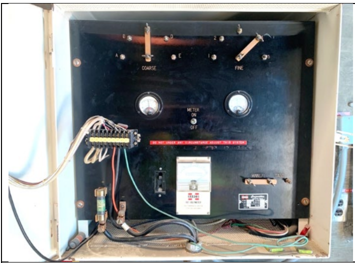
Photo: Impressed Current Rectifier
