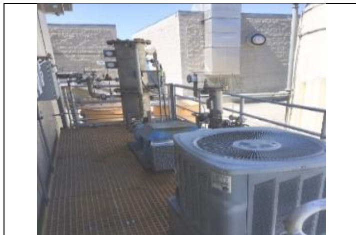
Photo: Existing Gas Conditioning System
