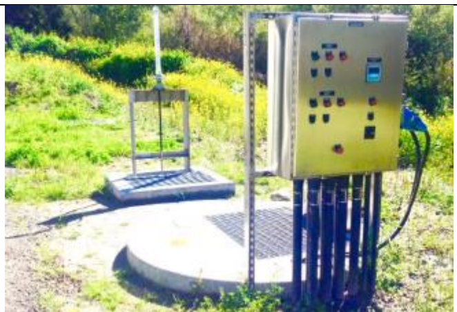
Photo: WWTP Stormwater Pump Station
