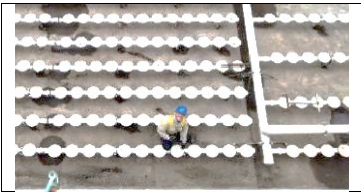
Photo: Existing air diffuser system
