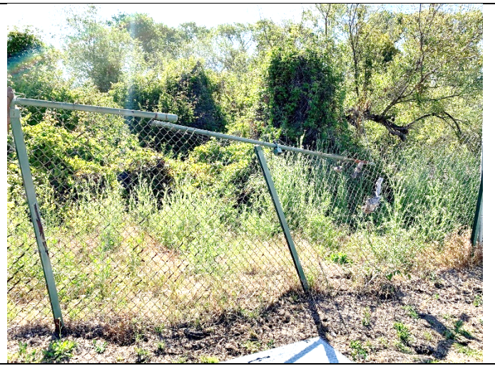
Photo: Existing Dilapidated Fence
