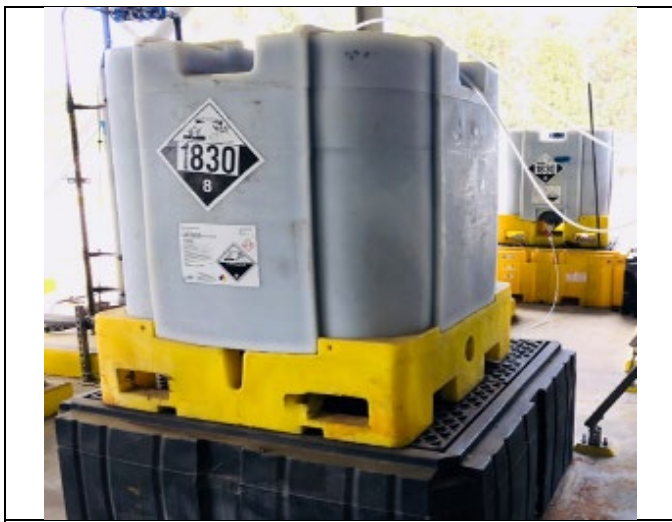
Photo: Existing totes used for Sulfuric Acid storage and Feed
