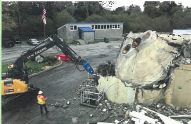
CAWD's circa-1930s digester was demolished in January to make way for new construction. We were able to get an amazing 85 years of service from the structure by converting it to a sludge holding tank after it had outlived its useful life.
