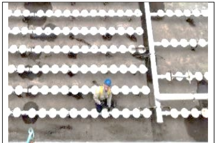
Photo: Existing air diffuser system
