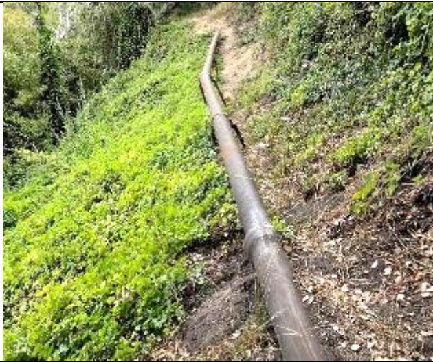
Photo: Sagged Pipeline
