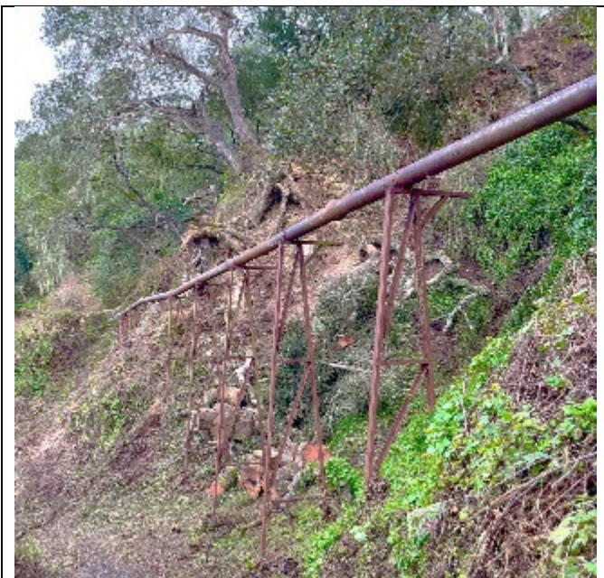
Photo: Aerial gravity pipe in easement
