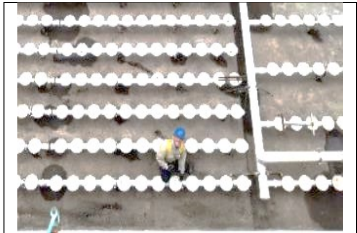
Photo: Existing air diffuser system
