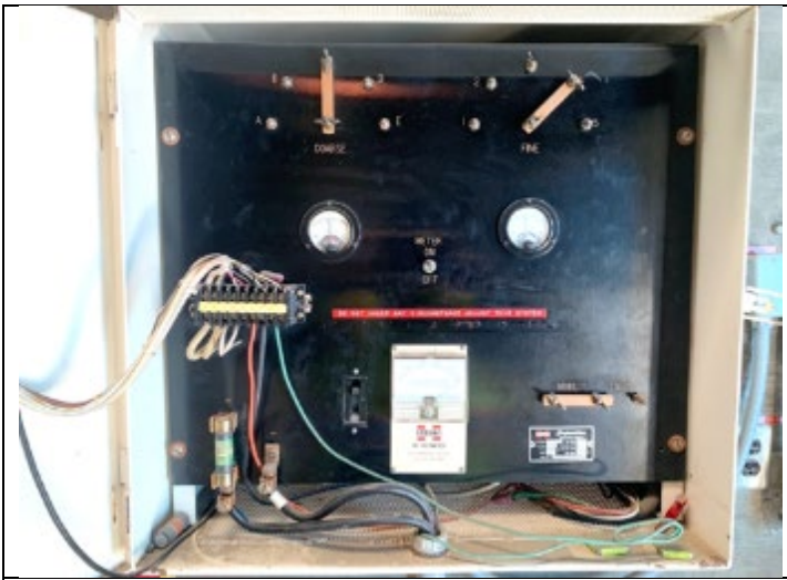
Photo: Impressed Current Rectifier
