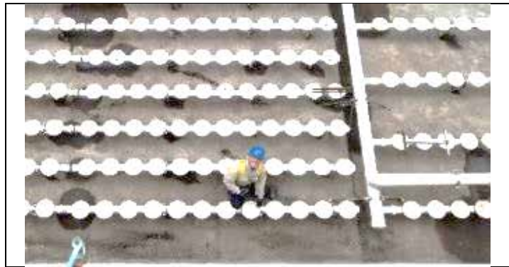
Photo: Existing air diffuser system
