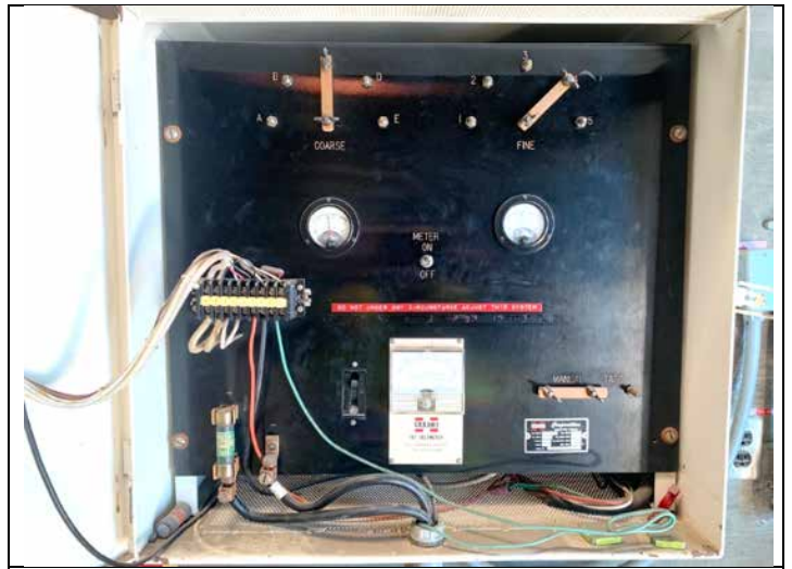
Photo: Impressed Current Rectifier
