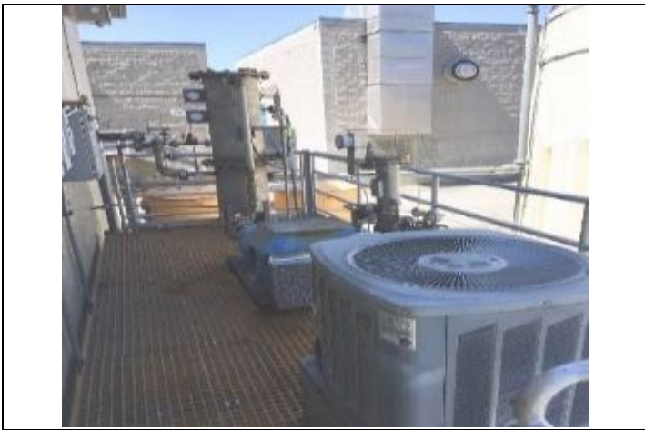
Photo: Existing Gas Conditioning System
