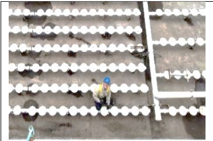
Photo: Existing air diffuser system
