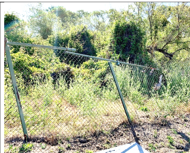
Photo: Existing Dilapidated Fence
