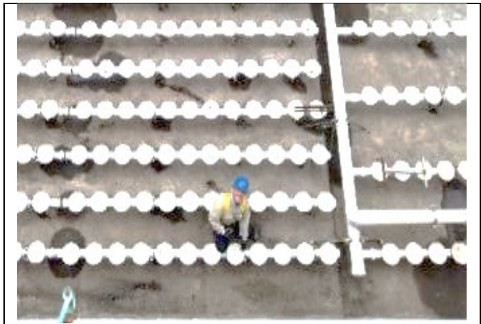
Photo: Existing air diffuser system
