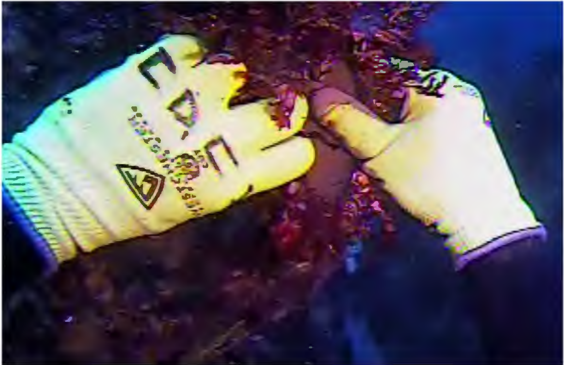
Image 2 – Duckbill contact sealing surface during no-flow (2021 image)
