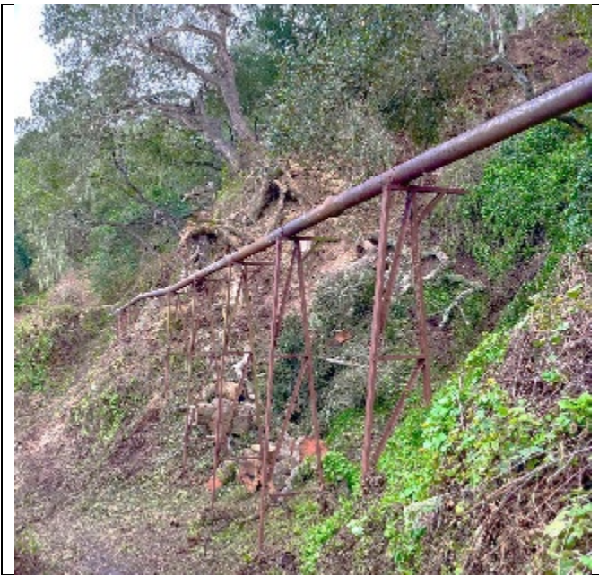
Photo: Aerial gravity pipe in easement
