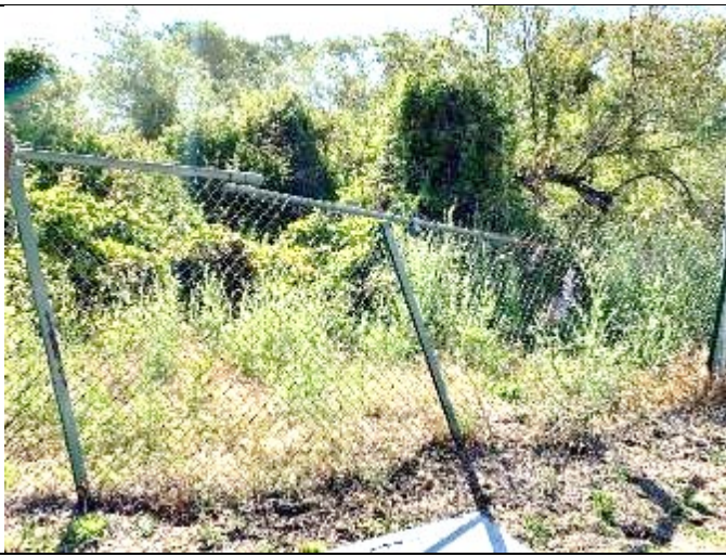
Photo: Existing dilapidated fence
