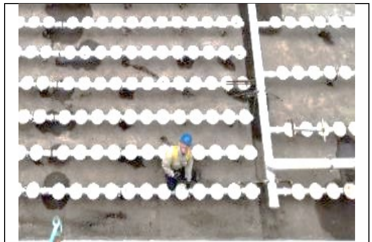
Photo: Existing air diffuser system
