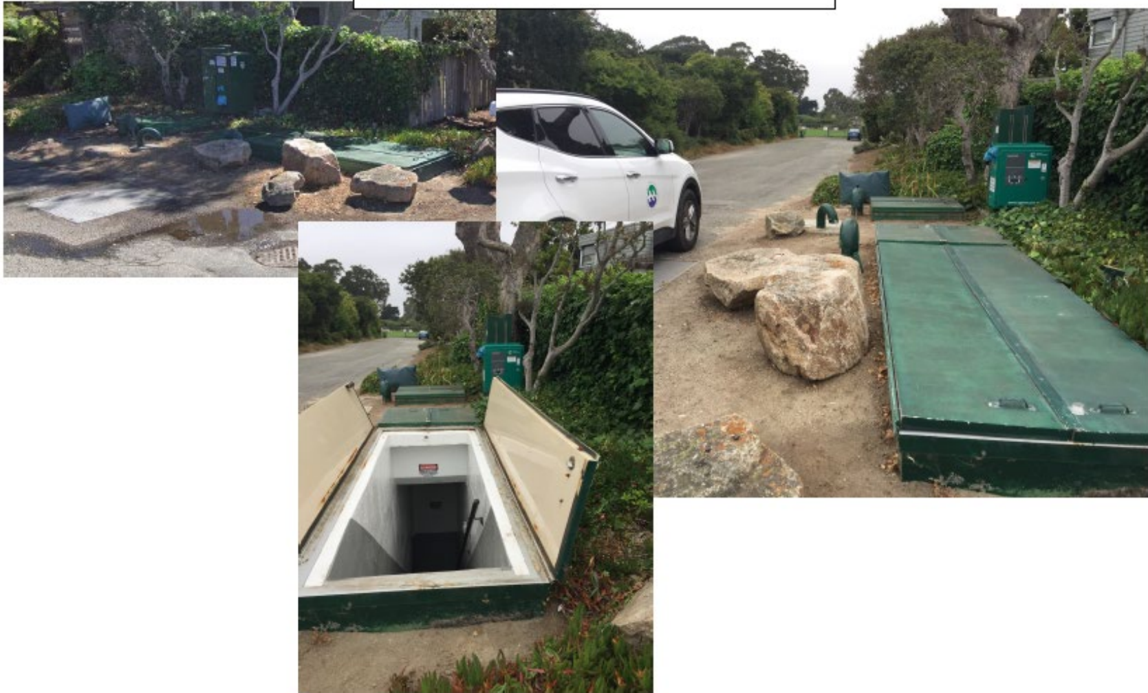
CAWD – Monte Verde and Sixteenth Pump Station
