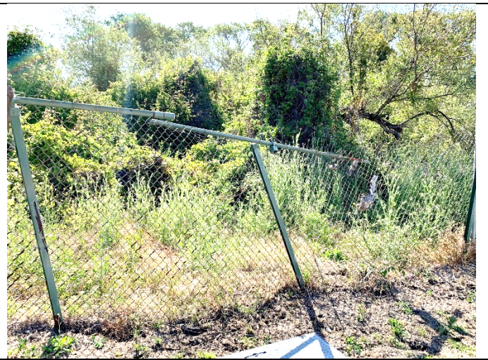
Photo: Existing Dilapidated Fence
