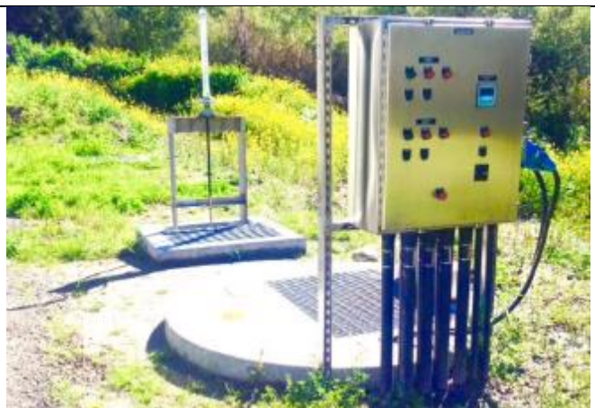
Photo: WWTP Stormwater Pump Station
