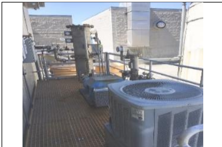
Photo: Existing Gas Conditioning System
