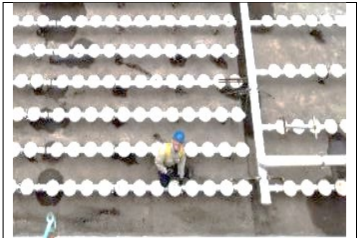
Photo: Existing air diffuser system
