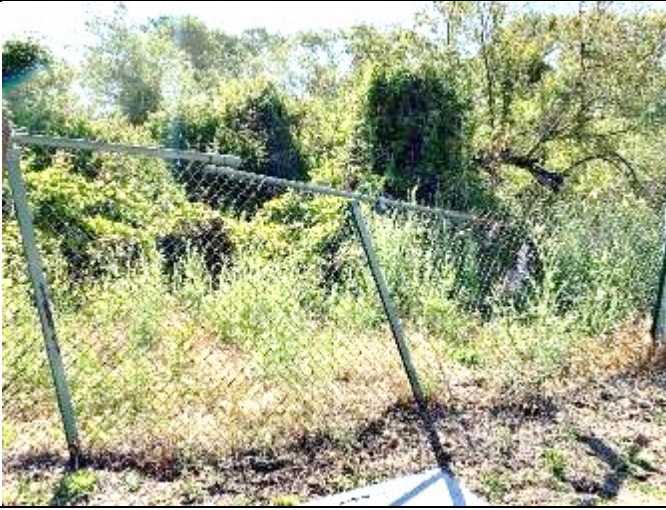
Photo: Existing dilapidated fence
