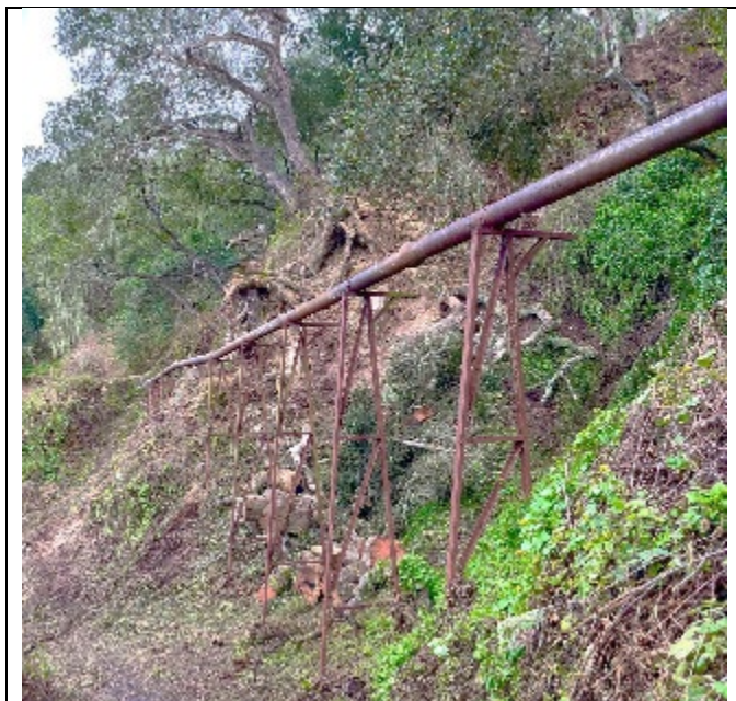
Photo: Aerial gravity pipe in easement
