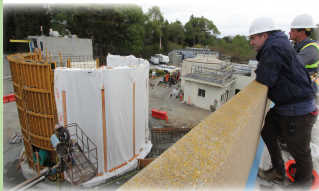
A TOPSIDE VIEW OF OUR COMMUNITY'S NEW SLUDGE HOLDING TANK CAWD's treatment plant renovation will be largely completed next year, on budget and ahead of time, to ensure public health and safety, and protect the local environment for the next 30? years.
