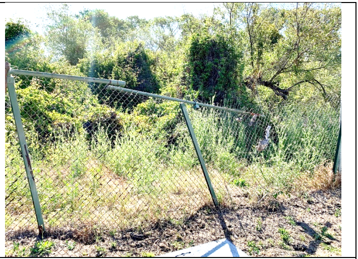
Photo: Existing Dilapidated Fence
