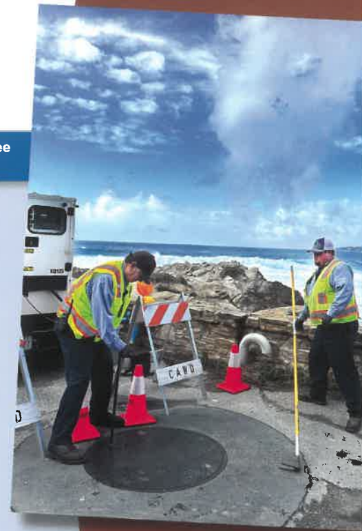
PRE-STORM PRECAUTIONS CAWD collections crew members prepare to inspect the wet well at our Scenic Road pump station before arrival of the February storms. The generator at left stands ready to provide immediate backup power during outages.
