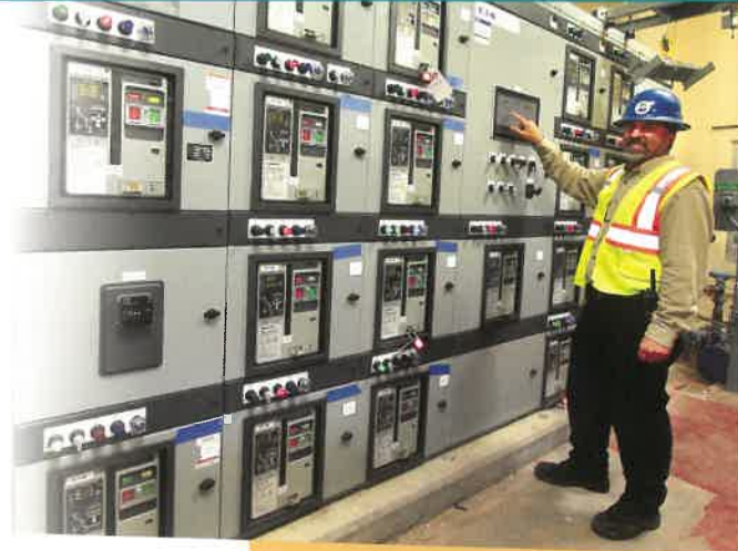
Senior Operator Christian Schmidt checks the status monitor on CAWD's new motor control center, which provides power for all pumps and motors at the treatment plant. Equipment upgrades installed as part of our 15-year master plan have helped reduce power costs by approximately 15 percent.
