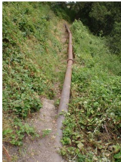
Photo 6 Reach 4 Facing northwest – outward rotation of foundation support
