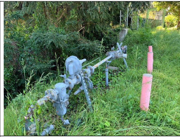
Photo: Gas Meter on North Side of River
