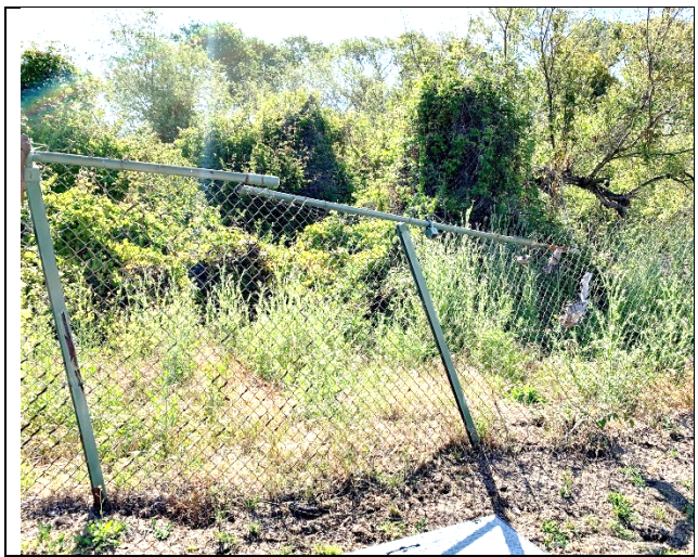
Photo: Existing Dilapidated Fence
