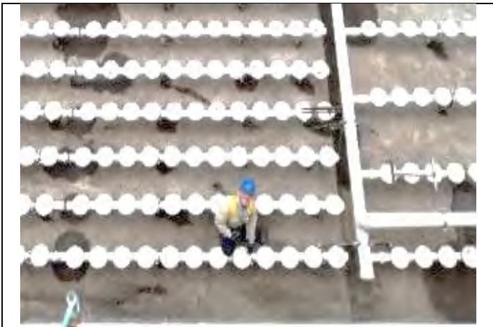
Photo: Existing air diffuser system
