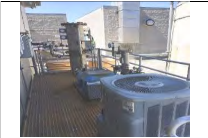
Photo: Existing Gas Conditioning System
