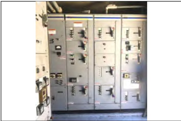
Photo: Existing Headworks Motor Control Center to Be Replaced in Project
