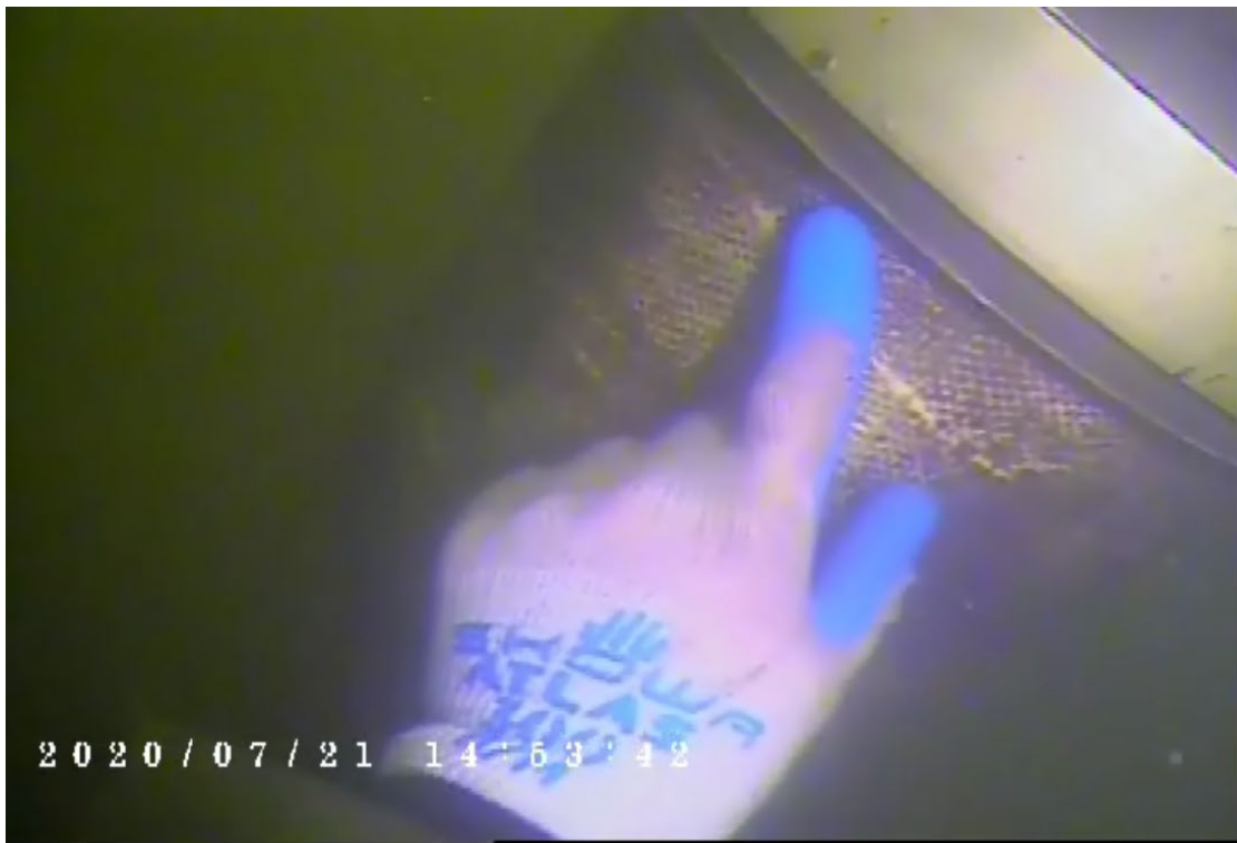
Image 6 – Lower epoxy and woven fiber wrap treatment with two-part clamp and rubber liner (typical)
