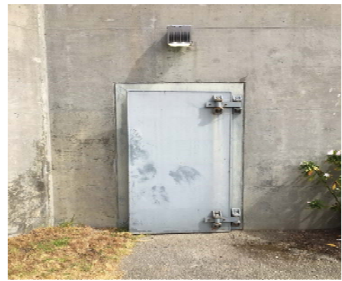
Photo: Old Flood Door in Headworks Basement
