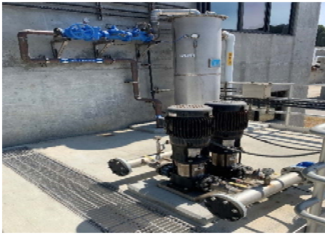
Photo: New #1 Water System where Corrosion System Project will be Installed
