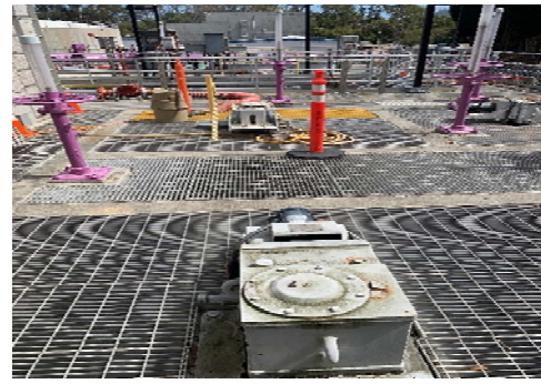
Photo: Existing Coagulation/Flocculation System and Sand Filters
