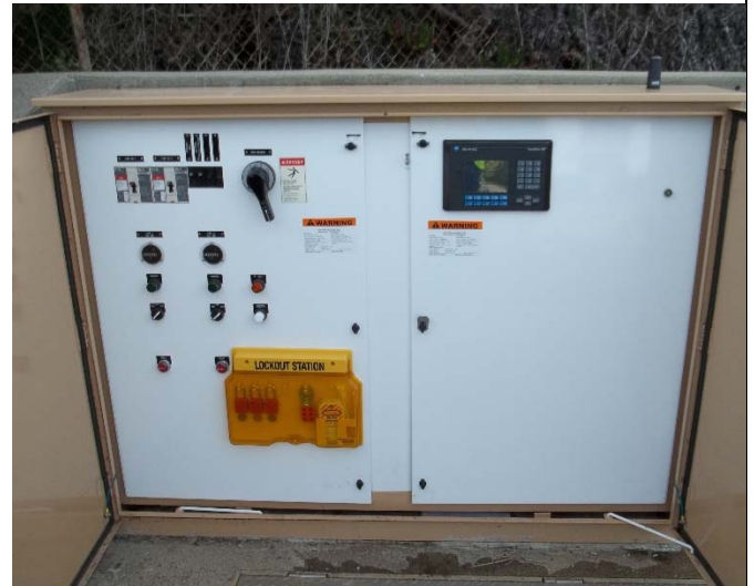
Photo: Pump station Control Panel- PLC and Operator Interface will be upgraded at Pump stations.
