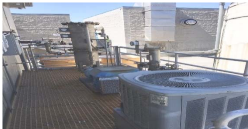
Photo: Existing Gas Conditioning System
