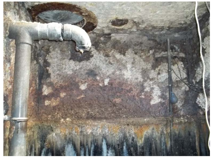
Photo: View H2S damage to Calle La Cruz wet well
