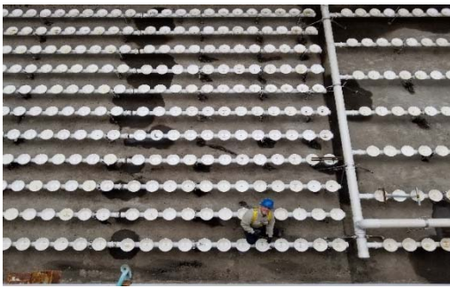
Photo: Existing air diffuser system
