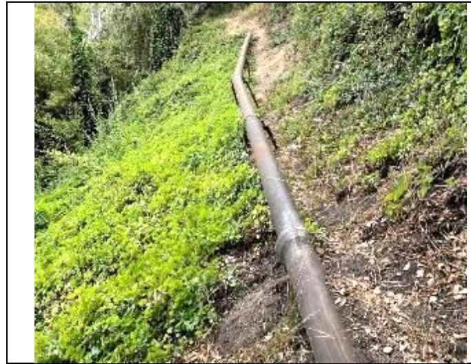
Photo: Sagged Pipeline
