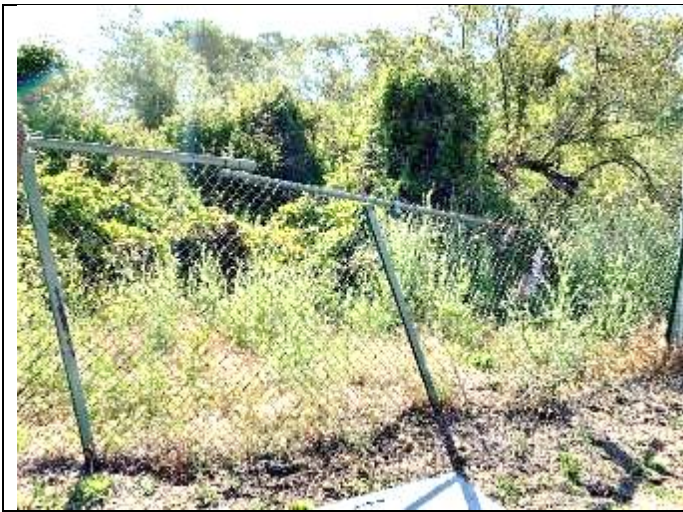
Photo: Existing dilapidated fence
