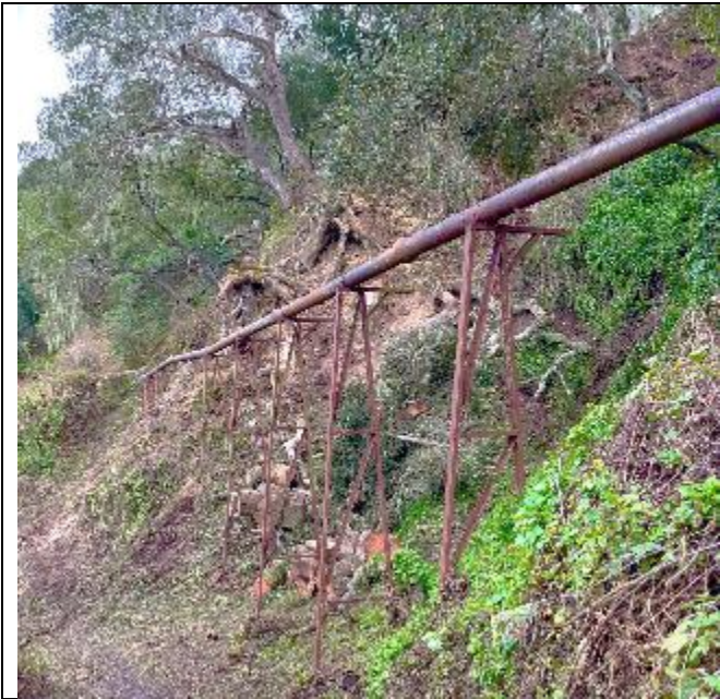
Photo: Aerial gravity pipe in easement
