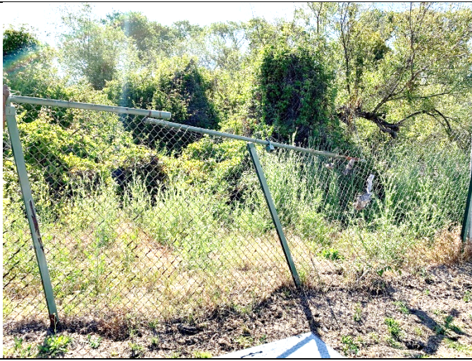
Photo: Existing Dilapidated Fence
