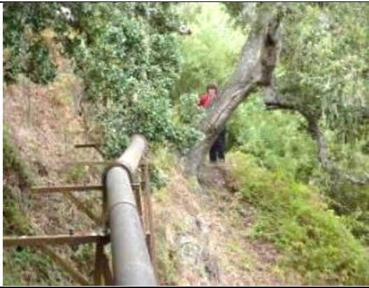
Photo: View gravity pipe in Carmel easement
