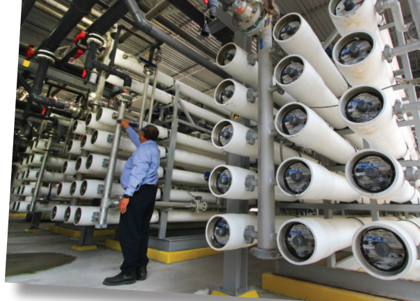
Disinfection destroys any viruses or pathogens that might remain in CAWD effluent after primary and secondary treatment. After that, treated wastewater undergoes another tertiary filtration before entering our cutting-edge microfiltration/reverse osmosis system (shown there), which produces pristine recycled water for irrigation.
